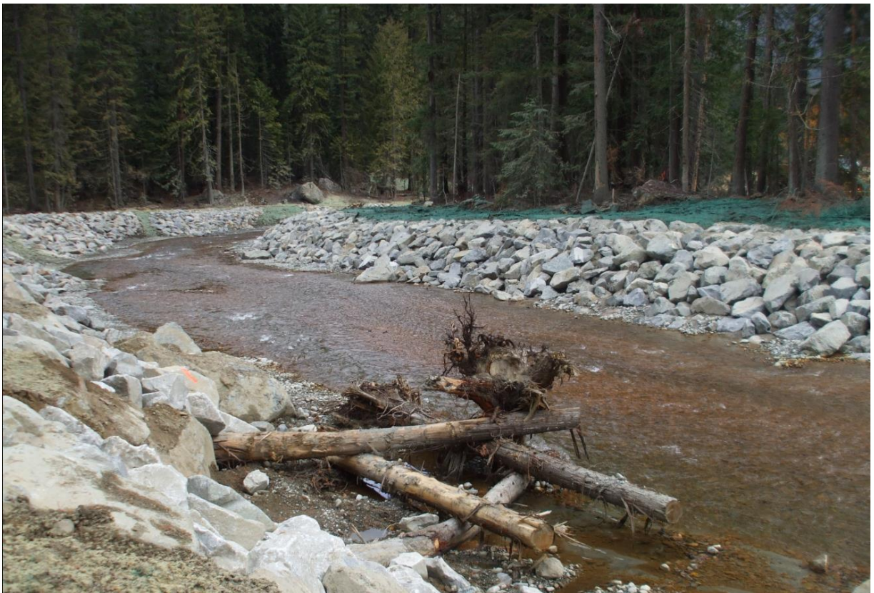
Railroad Creek segment 1, Nov. 1, 2013. Water now flows into the new alignment. The disturbed areas along banks of the Railroad Creek realignment area received seed and hydro mulch, along with other winterization measures.
