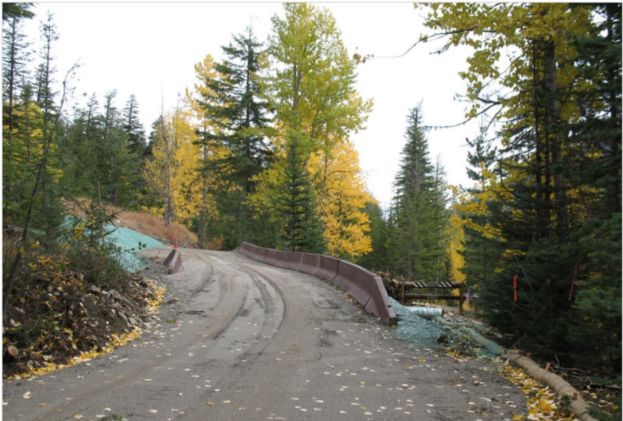
New road at Holden ball field. A new road was developed to access the ball field just beyond Holden Village area which will be used as a storage and staging area during heavy construction.
