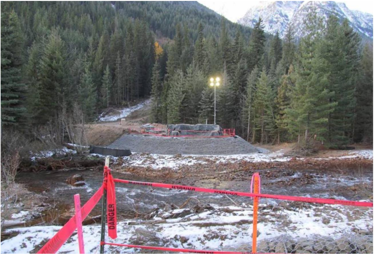
A temporary bridge over Railroad Creek was put in place as part of the bypass road to the mine site. The bypass road was constructed to minimize construction traffic through Holden Village.
