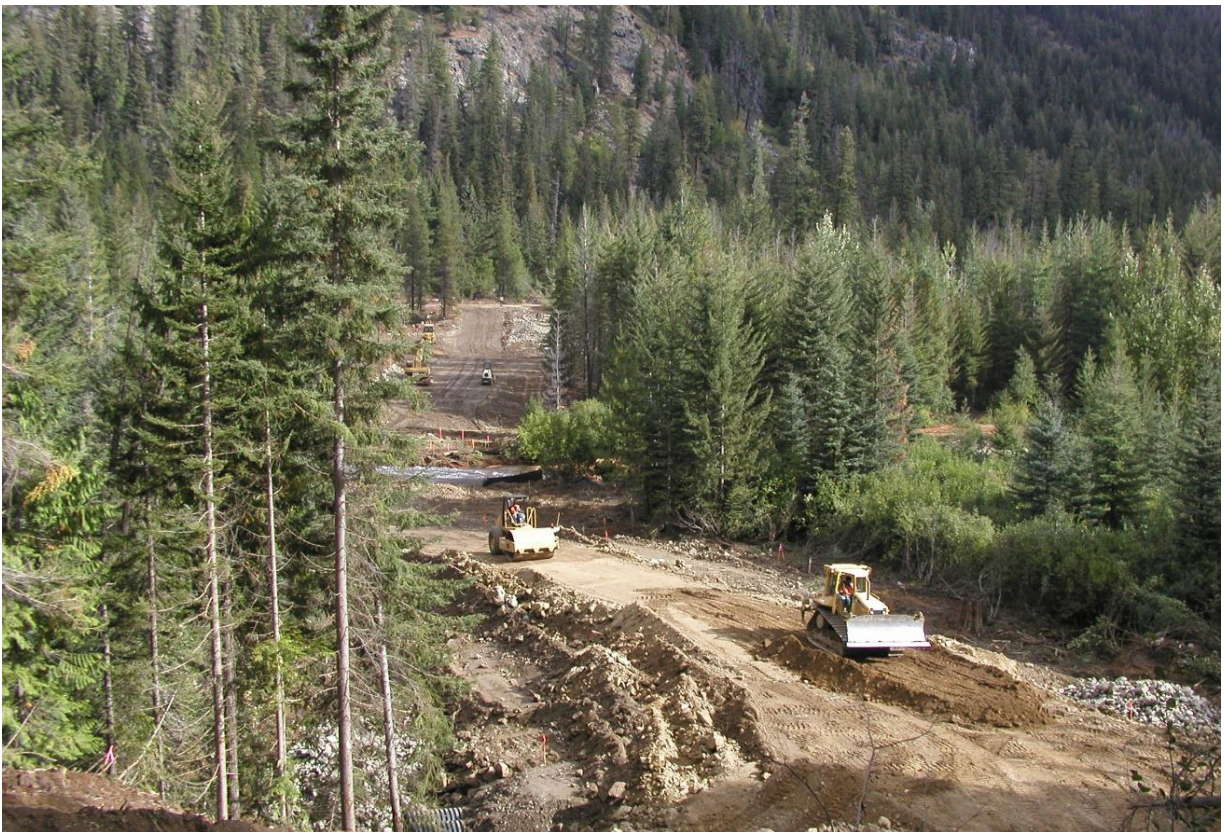
East bypass road crossing and prepping of the bridge location. Looking northeast at the prep work for the temporary bridge over Railroad Creek.
