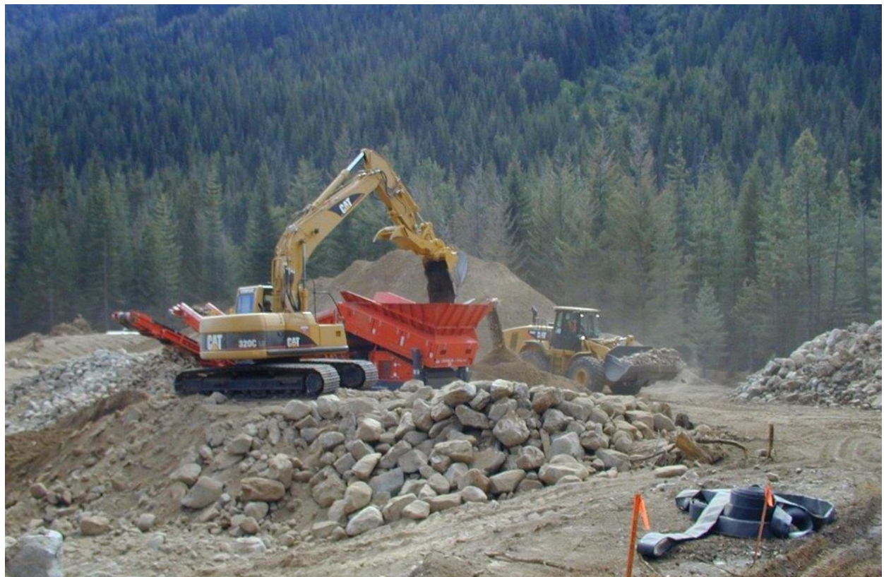
Lower West Ten Mile Borrow is one of three sites where rock, gravel, and soil is collected.
