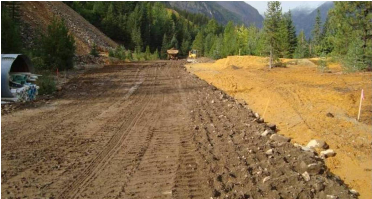
Bypass road construction, tailings and bypass. To access the mine site, the bypass road travels over tailings pile 1 and tailings pile 2 (orange material in the picture).
