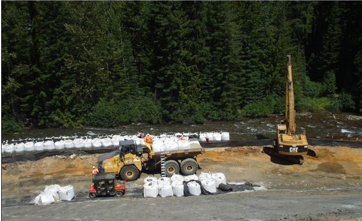
Super sacks in Railroad Creek, June 2013. Large bags filled with sand, also known as "super sacks", were used to divert the creek water away from the stream bank so the barrier wall platform could be constructed.
