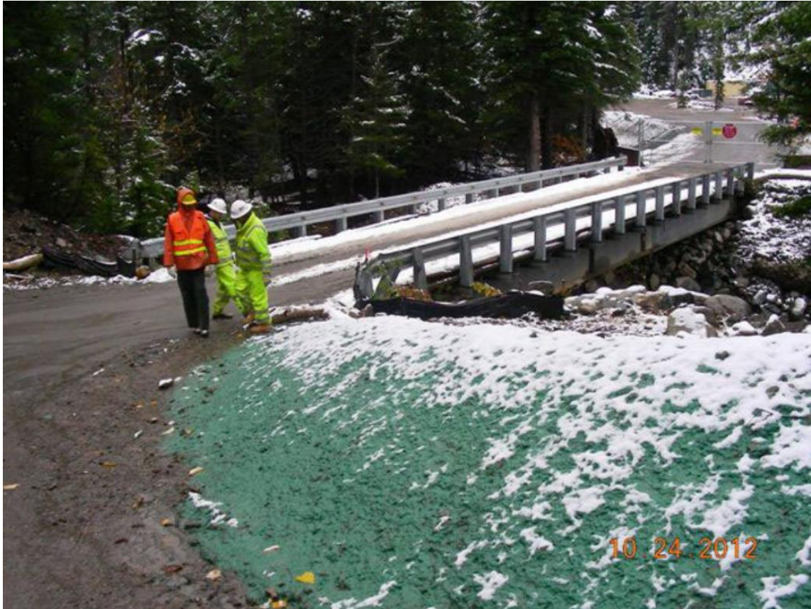
Areas along the Holden bypass road and Forest Service Road 8301 received hydro seeding to encourage vegetation growth in the spring. 10-24-2012.
