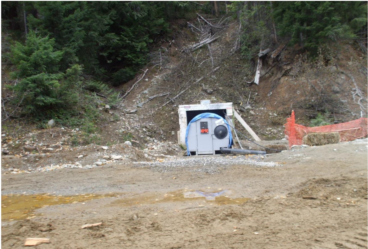
Main portal, Nov. 1, 2013. To capture water draining from the underground mine workings, crews completed constructing concrete bulkheads in the Main and Ventilator Portals.
