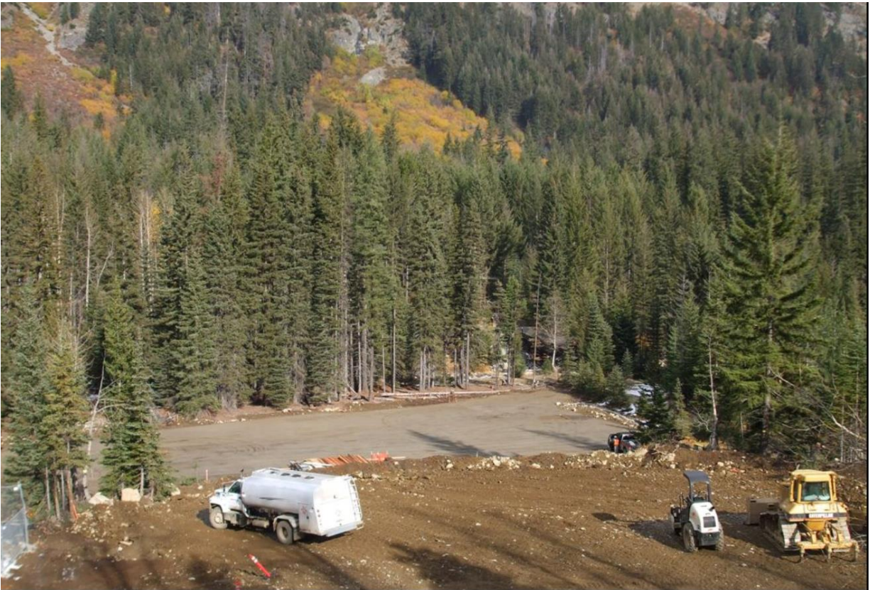
Staging area. This area was prepped as a staging area for temporary contractor facilities.
