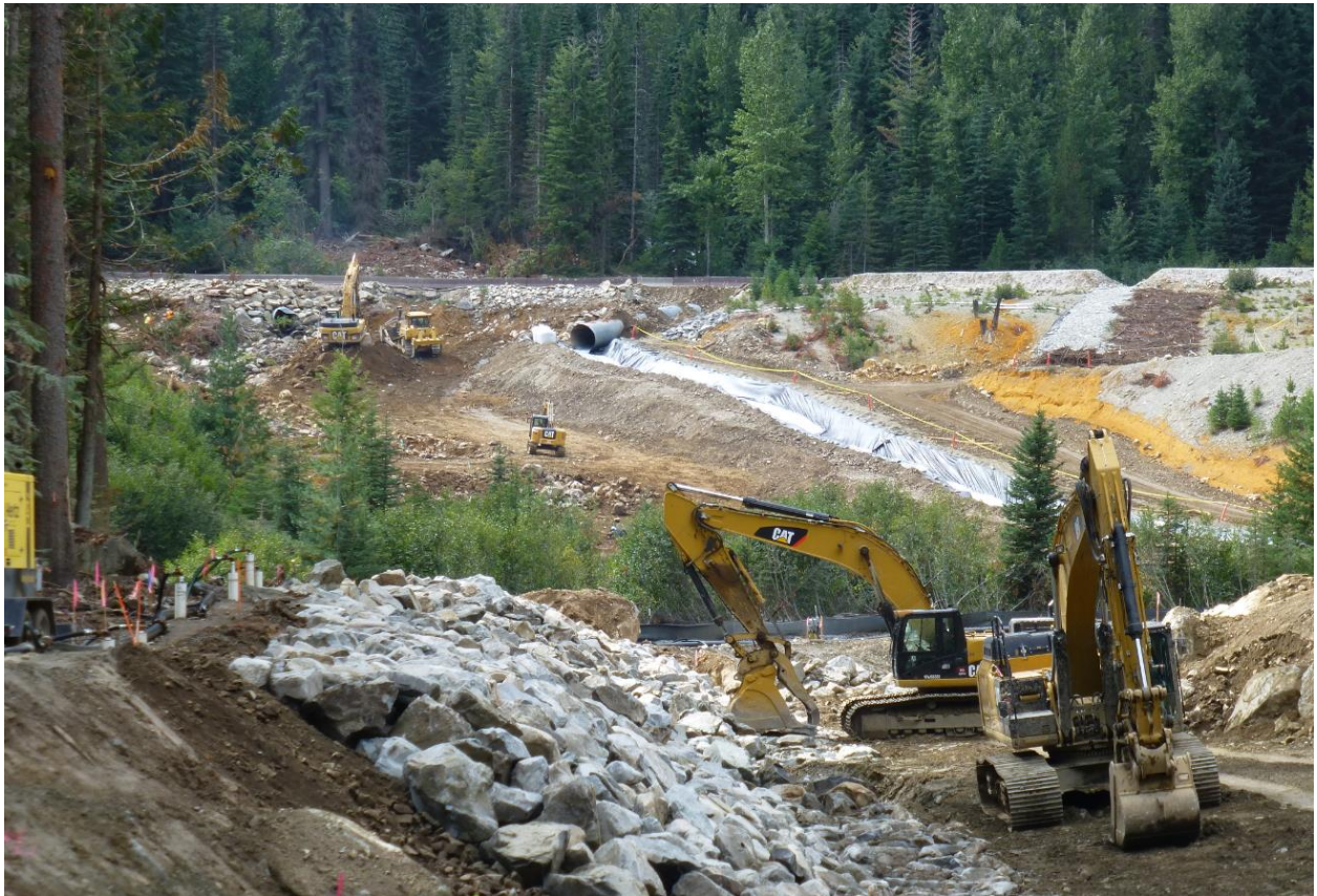
Railroad Creek Construction placing rock in creek bed. Development of Railroad Creek.
