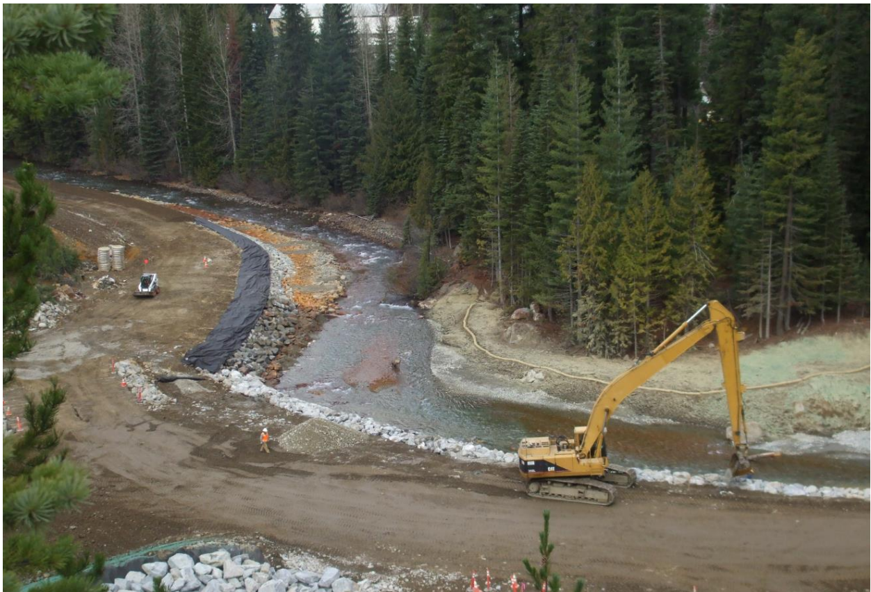
Barrier wall platform below tailings pile 1, Nov. 1, 2013. The barrier wall platform is in the process of being constructed from east of tailings pile 1 along Railroad Creek and past the toe of tailings pile 2. This platform lays the foundation for the below grade barrier wall that will be installed during the 2014 field season.
