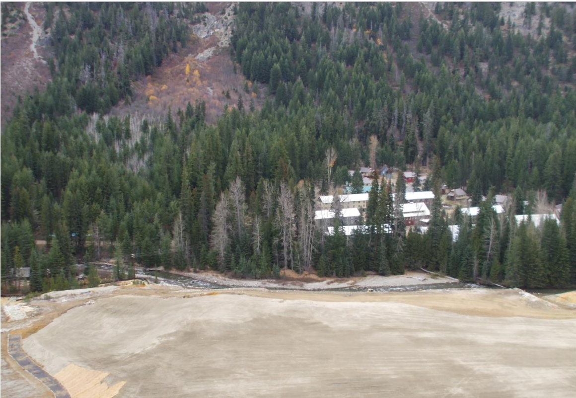
Grading of Tailings Pile 1, Nov. 1, 2013. Contractors finished grading Tailings Pile 1 for the 2013 construction season. The grading involved utilizing an excavator to load trucks and haul the tailing to Tailings Pile 3 to be spread and compacted. A temporary cover was placed over the newly graded Tailing Pile 1.
