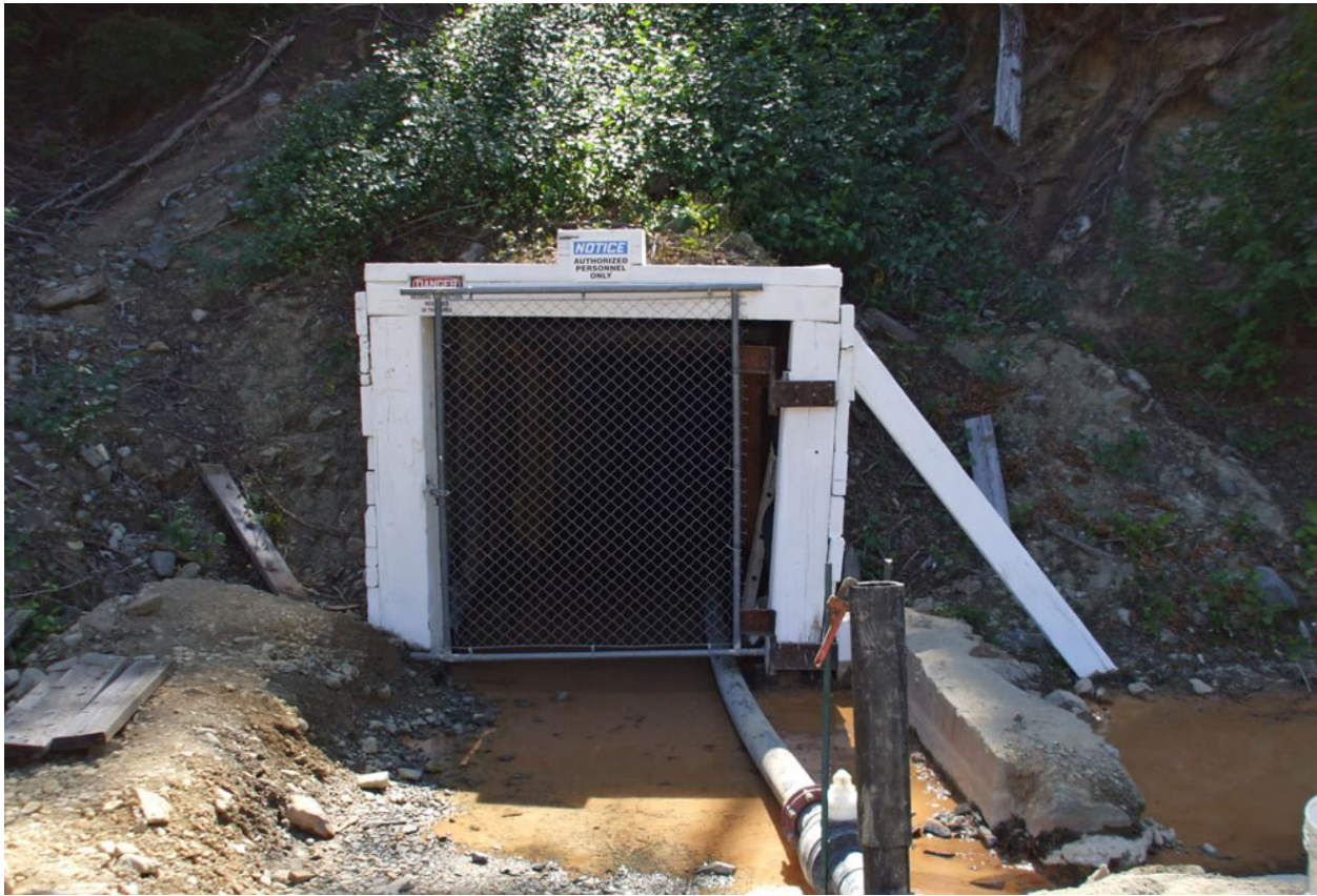
Main Portal--stabilization and sealing of the old entrances to the underground mine so mine drainage can be controlled and treated.
