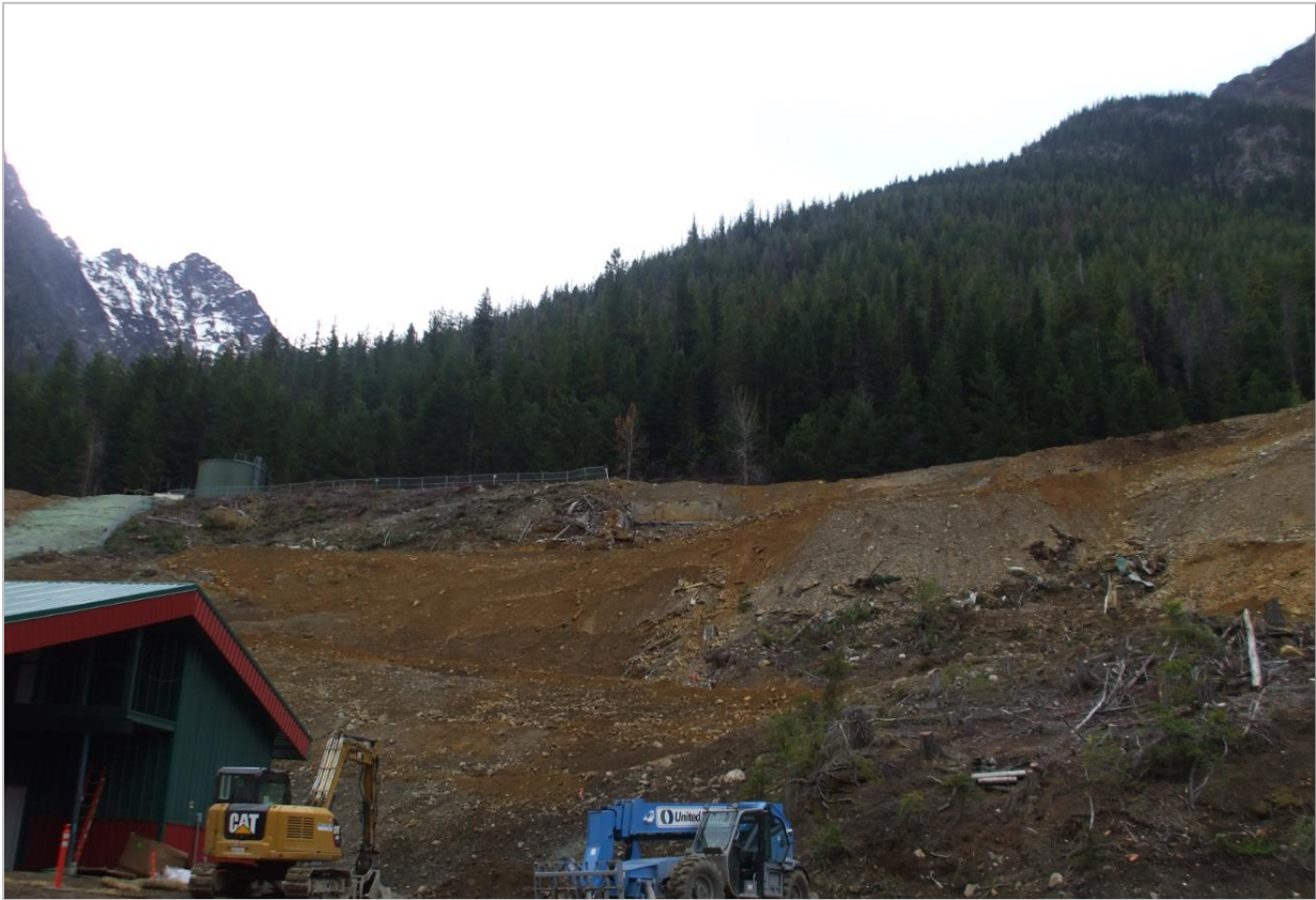
Previous mill structure location, Nov. 1, 2013. The superstructure of the Mill has been dismantled. Excavators with hydraulic hammer attachments were used to demolish concrete, while excavators and articulated trucks removed demolition debris from the work area. A bench was prepared for placing demolition debris within the former Mill structure area. The demolition debris was then returned to the Mill structure footprint, covered and compacted with waste rock.
