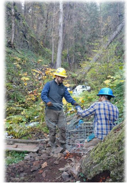
Crews creating gabions for the new bridge on the Wahkeena Falls Trail
