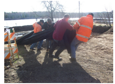
Alger County Road Commission employees are excited about how their Recovery Act project will benefit the local community. Surveying the work in progress, ACRC Foreman, Dave Maki, and his crew, put it this way: "When we get done here, this facility is going to be really nice for local people and visitors to use."
