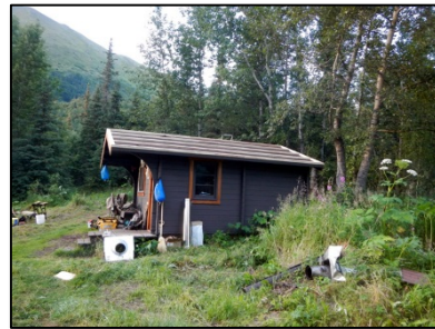
Swan Lake Cabin in progress of getting a new roof and chimney system.
