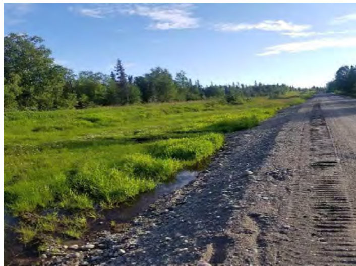
Figure 49. Young reed canarygrass in a low lying, wet area of the North Road Extension/Pipeline Access ATV trail construction zone. Courtesy photo by Maura Schumacher.
