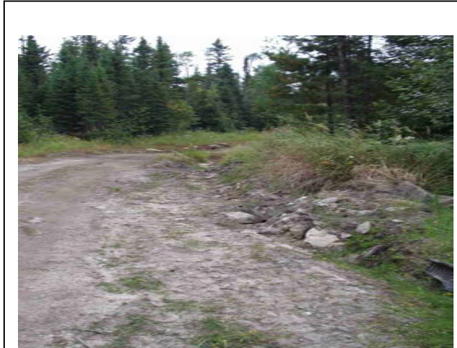
Little East Creek Access trail –after (Sept 2005) Fill brought in, smoothed site, grassing in.
