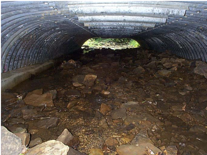
Figure 5. Illustrates an open bottom arch culvert that maintains the natural substrate, and allows for passage of all aquatic species.
