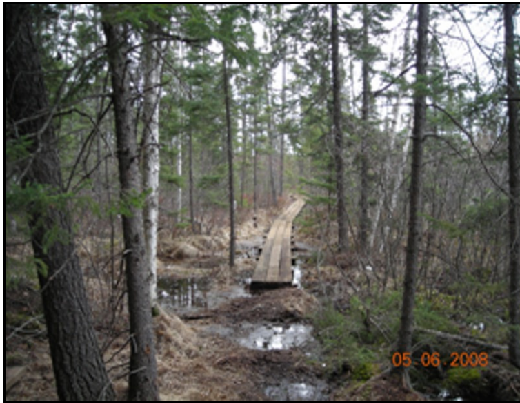
Figure 3.1. Pear Lake boardwalk constructed to facilitate access to Pear Lake across a wetland while preventing damage to the wetland on the Superior National Forest.
