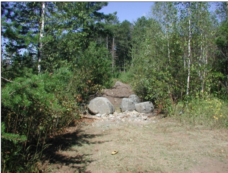
Figure 14.1 Immediately (2007) after decommissioning a road on the Nira Project 13 on the Superior National Forest.
