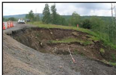
Slope failure in Highway 65 on Grand Mesa
