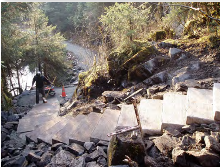
Installation of concrete steps at the Trail of Time. Photos by Peter Cross.
