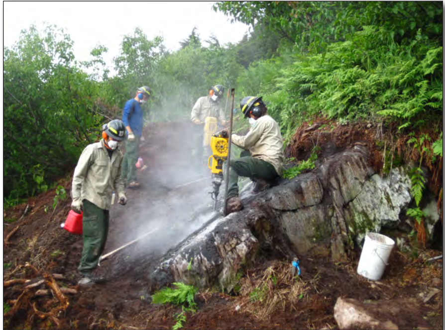
Glacier trail crew members Ari Stiassny, Shane Patrick, Kent May, and Cody Knoop drill rock along the Glacier Discovery Trail. Photo by Tony Fiorino.
