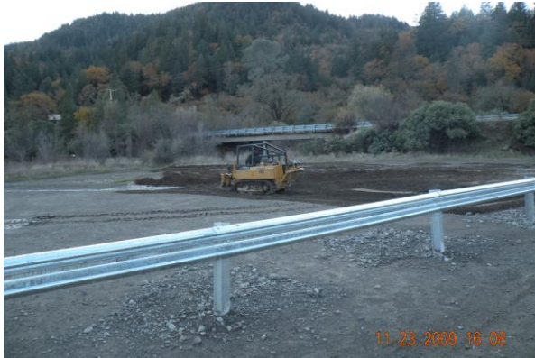
Photo 1 (Before): Picture is taken looking toward the Elk Mountain Rd bridge over the West Fork of Middle Creek. In the foreground is the OHV riding area being subsoiled to alleviate compaction. The highly compacted riding area would contribute significant amounts of runoff and fine sediment into the West Fork during even frequent low-intensity rainfall events.
