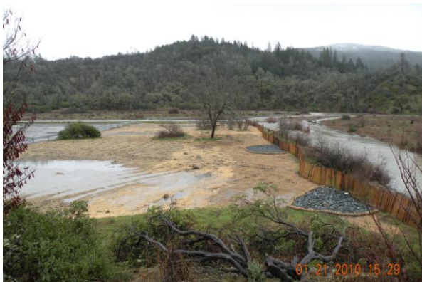
Photo 2 (During): Picture was taken from the bridge over West Fork Middle Creek the first winter after completion. Straw was used to stabilize the area until vegetation could take hold. Overland flow can be seen ponding in depressions allowing the majority of the runoff to infiltrate back into the soil and deposit fine sediments instead of spilling into West Fork. Also seen in this picture are two of the rocked outlets that were constructed for infrequent high-flow events. Rocked and waddled outlets also helped trap sediment. These outlets serve to also direct return flow back into the West Fork when it floods over its banks into the area.
