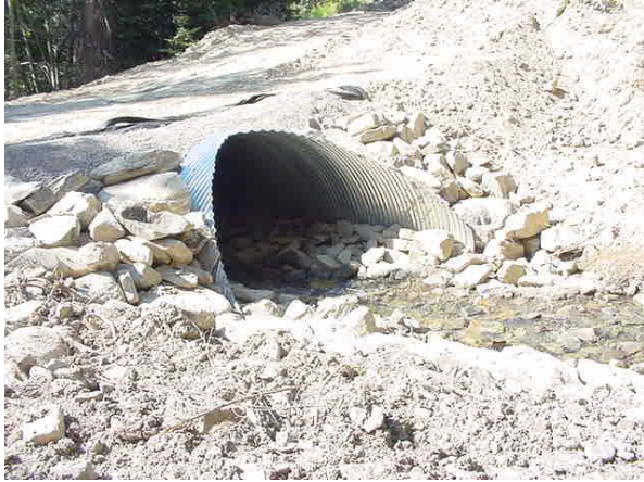
Figure 3. Counter-sunk pipe arch culvert. The stream channel is simulated through the crossing.
