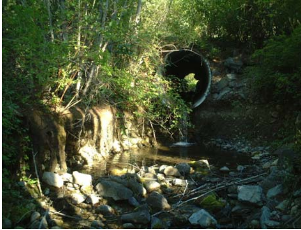
Figure 1. Bank undercutting at culvert outlet effectively preventing the passage of fish and other aquatic organisms.
