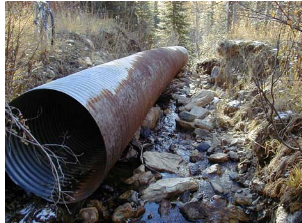
Figure 2. Culvert failure resulting from water piping.
