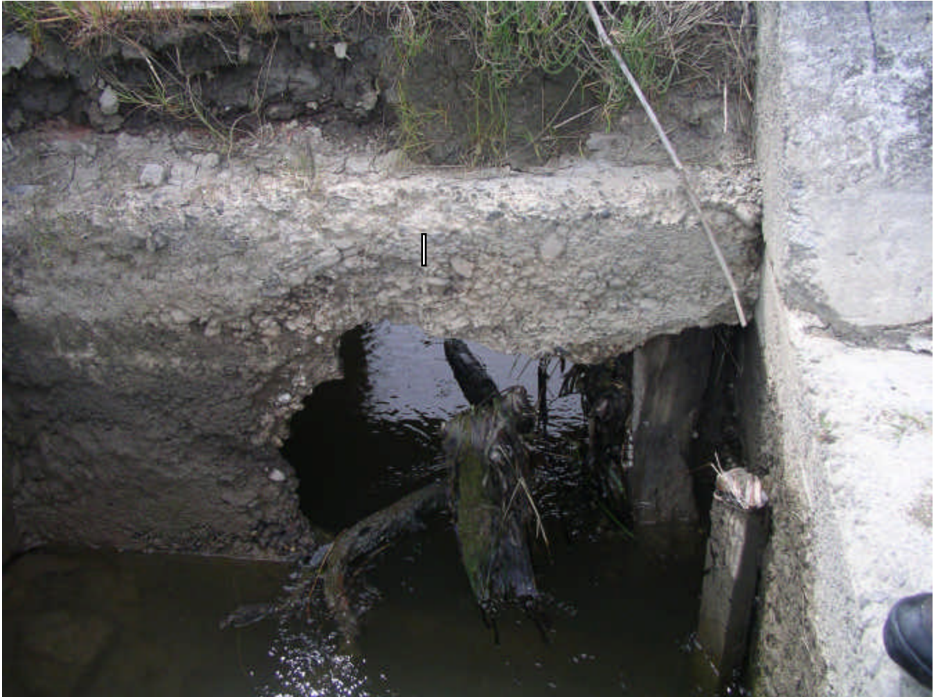
Figure 4. Photo showing the hole in the old tidegate headwall, with mud and debris cleared out.
