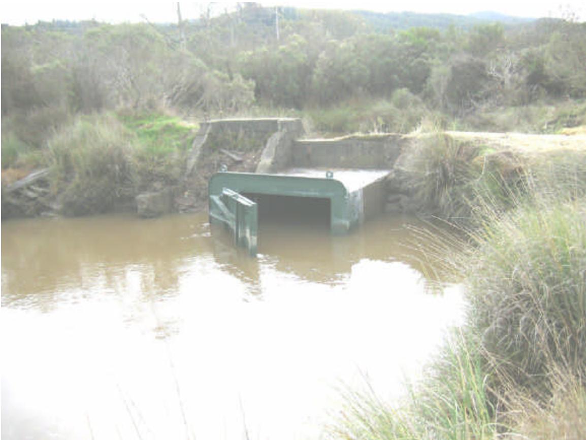
Figure 7. The completed tidegate project showing the tidegate open approximately one hour after the peak tide.
