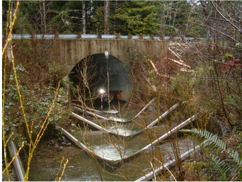
Figure 3-9. Peacock Ck (Tan Oak Dr, Del Norte Co, CA) vortex weirs can not be approximated as one-dimensional structures.
