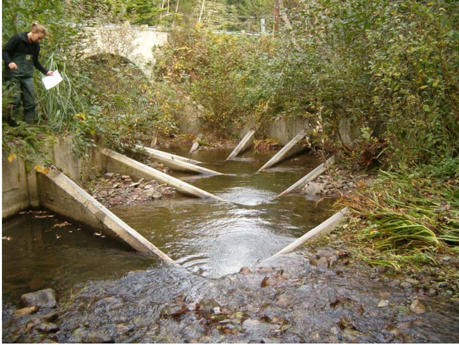
Figure 5-16. Peacock Creek field site. Looking downstream at vortex weirs at the upstream side of an arch culvert. The weir in the foreground is the most upstream weir in the series.
