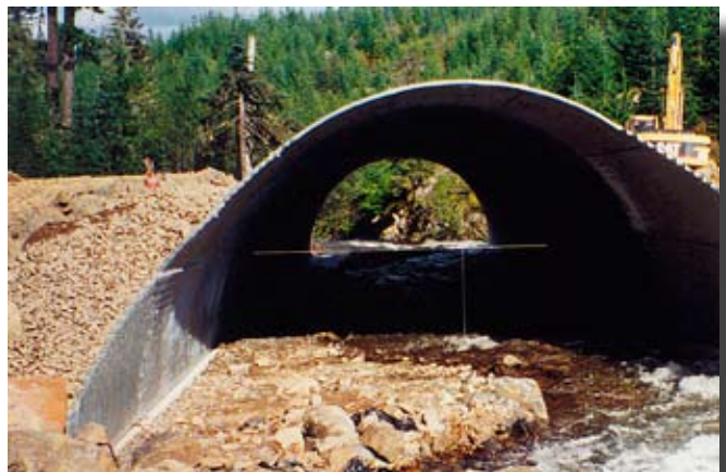
Figure 7.5—Multiplate open-bottom pipe arch.
