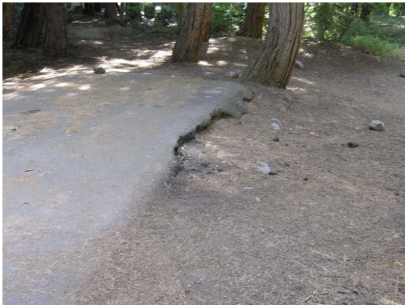
Figure 1-8. The camping spurs are very small and of variable sizes. The constrained size results in off-pavement parking and subsequent soil compaction and resource damage.
