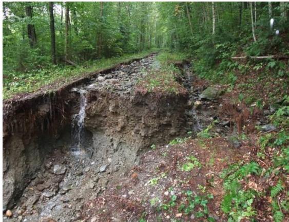
Boyden Brook Road and Trail Damage
