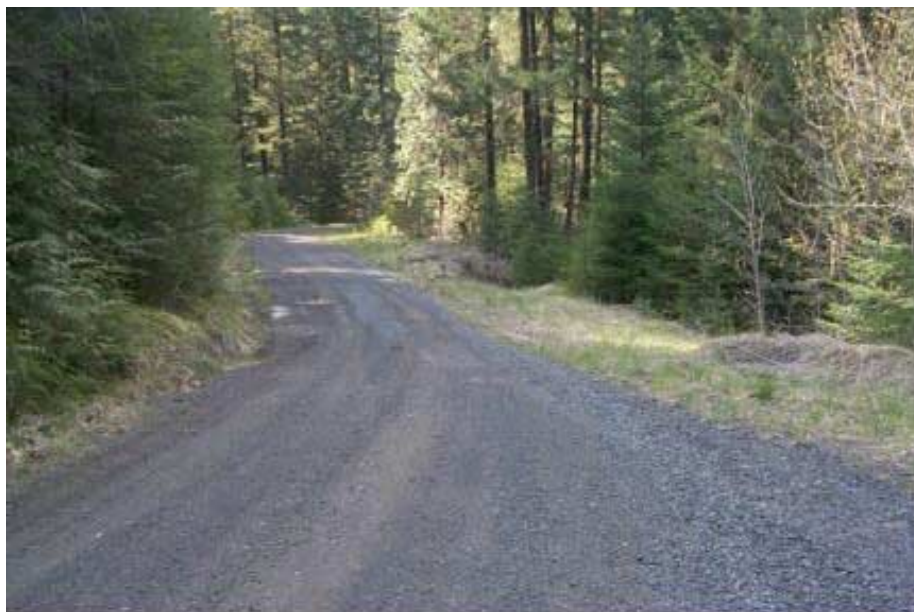
Figure 6—At the Willamette National Forest site, seasonal elevated pore water pressure has caused the road to sag several meters.
