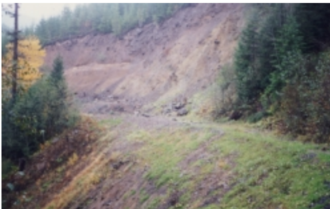
Figure 16—The largest slide on the Greenwater River Road removed 300 ft of roadbed in the inner gorge.
