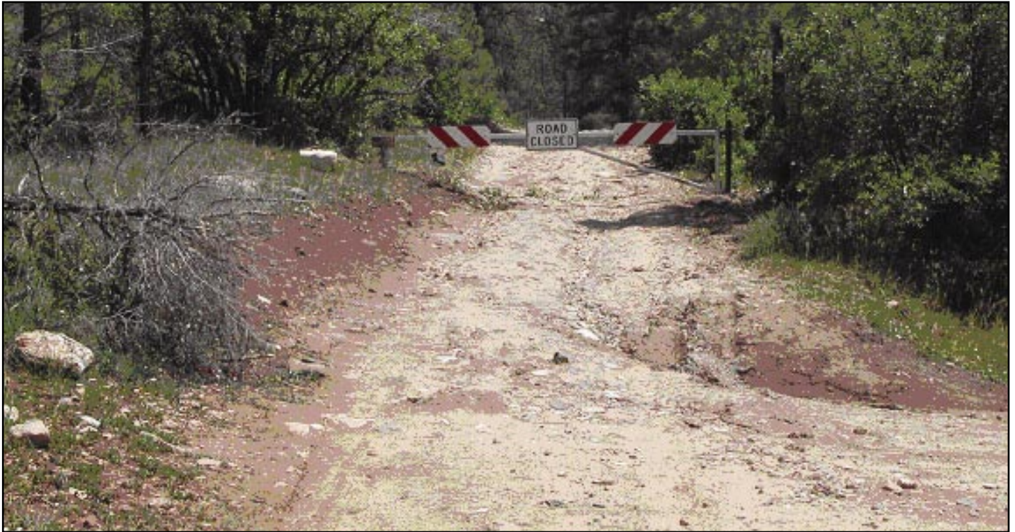
Figure 27—Maintenance level 2 road that has been “temporarily” closed.
