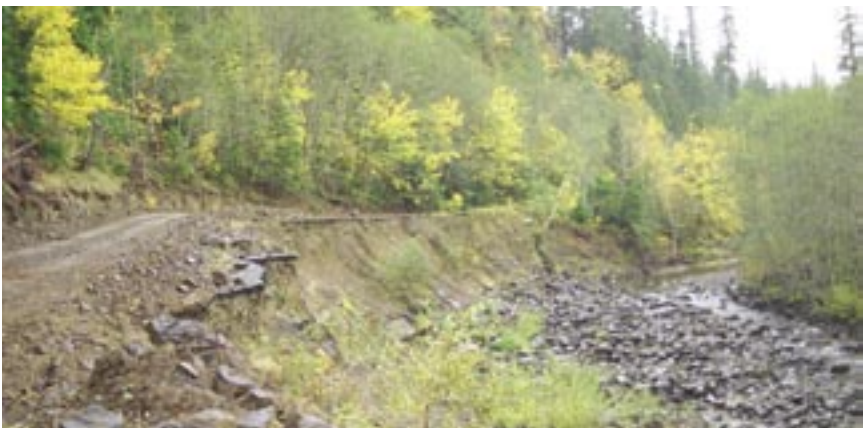
Road realignment needed.
