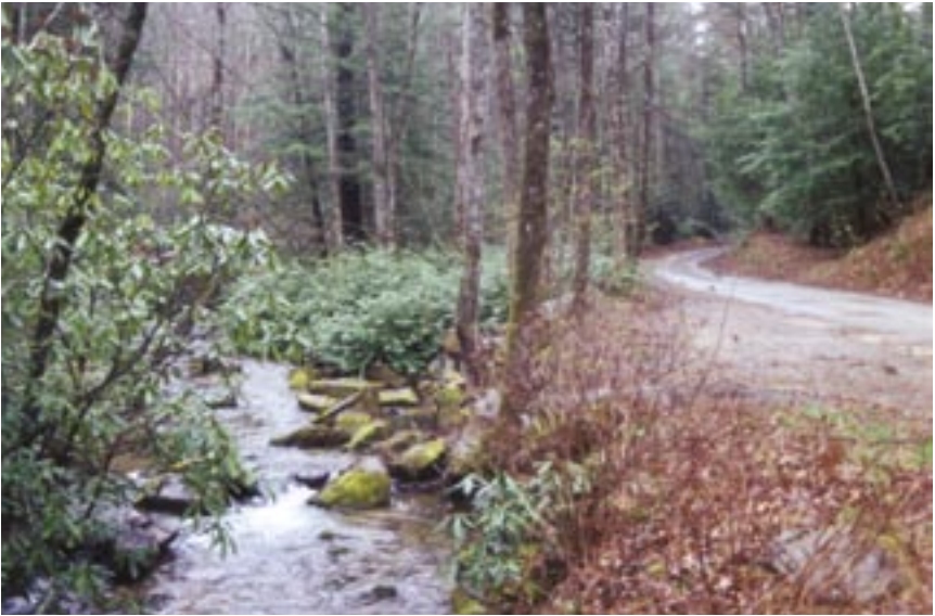
Road encroaching on riparian area.
