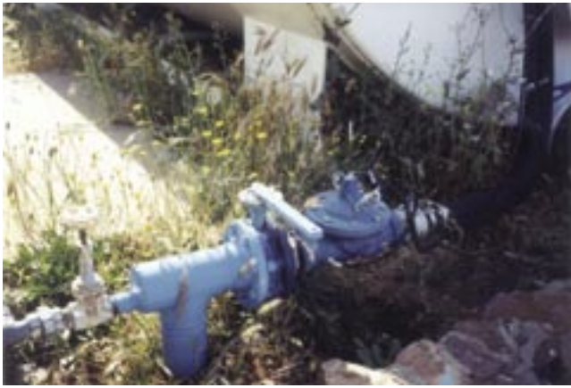
Figure 56—Automatic water valve.
