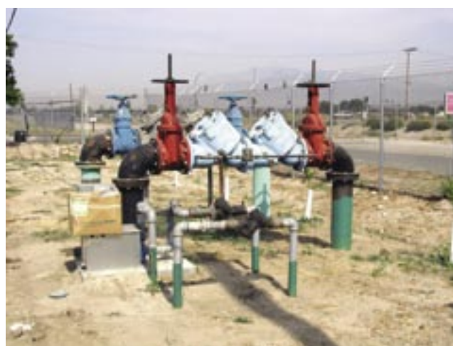
Figure 55—Backflow prevention valves.
