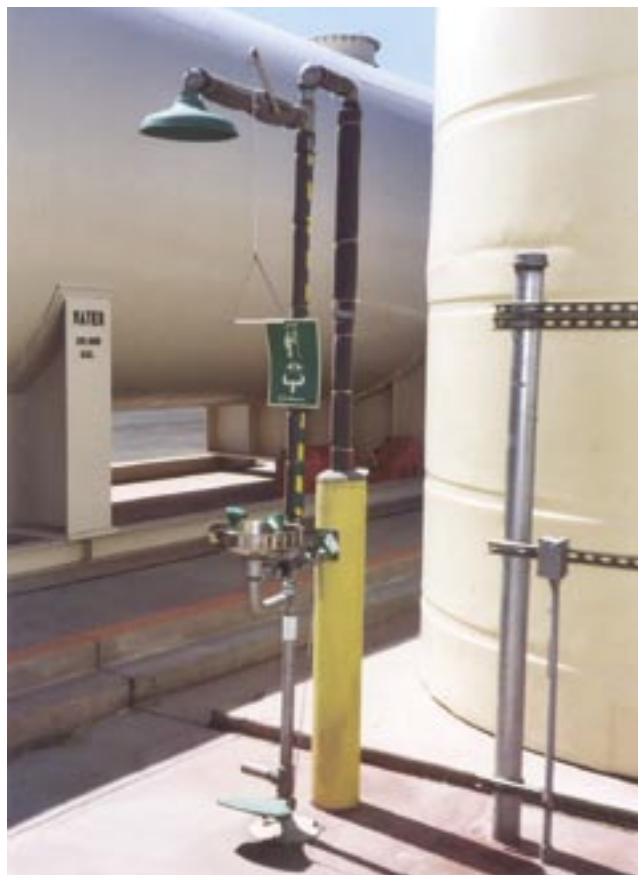
Figure 64—Emergency eyewash station (San Bernardino, CA).
