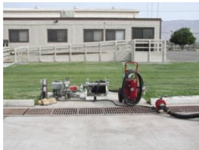
Figure 32—Loading pad utilities (San Bernardino, CA).
