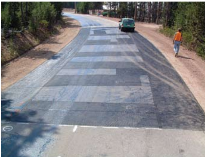
Figure 4—GlasGrid Type 8502 was used to treat the individual thermal cracks in test section 1. The darker areas are those covered by the GlasGrid.
