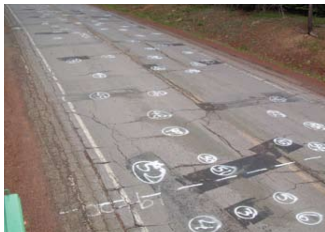
Figure 2—Test section 2, exhibiting a variety of pavement-cracking distress types.
