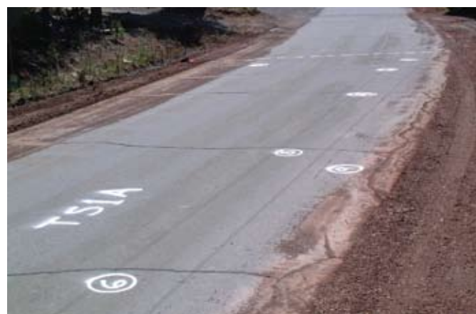
Figure 1—Test section 1, exhibiting large, regularly spaced thermal cracks.
