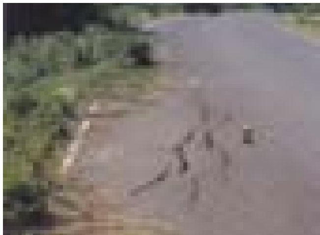
Figure 2—Pavement cracking as evidence of sidecast fill settlement.
