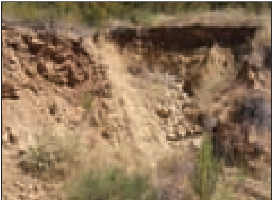
Figure 4—Typical gully erosion.
