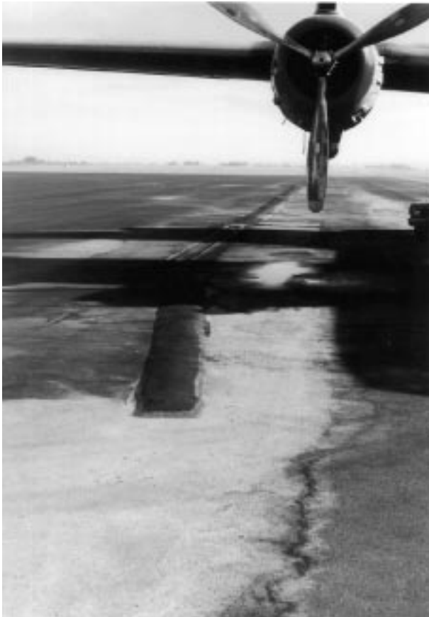
Figure 45. Asphalt Berm and Drain—Pocatello, ID.
