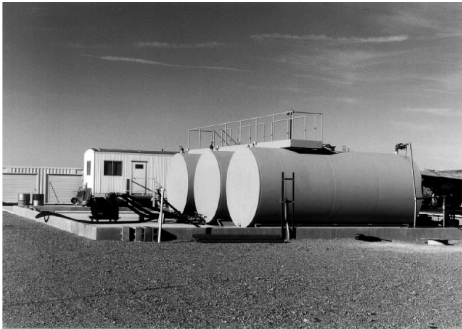
Figures 42 A&B. Tank Spill Containment Wall—Pocatello, ID.
