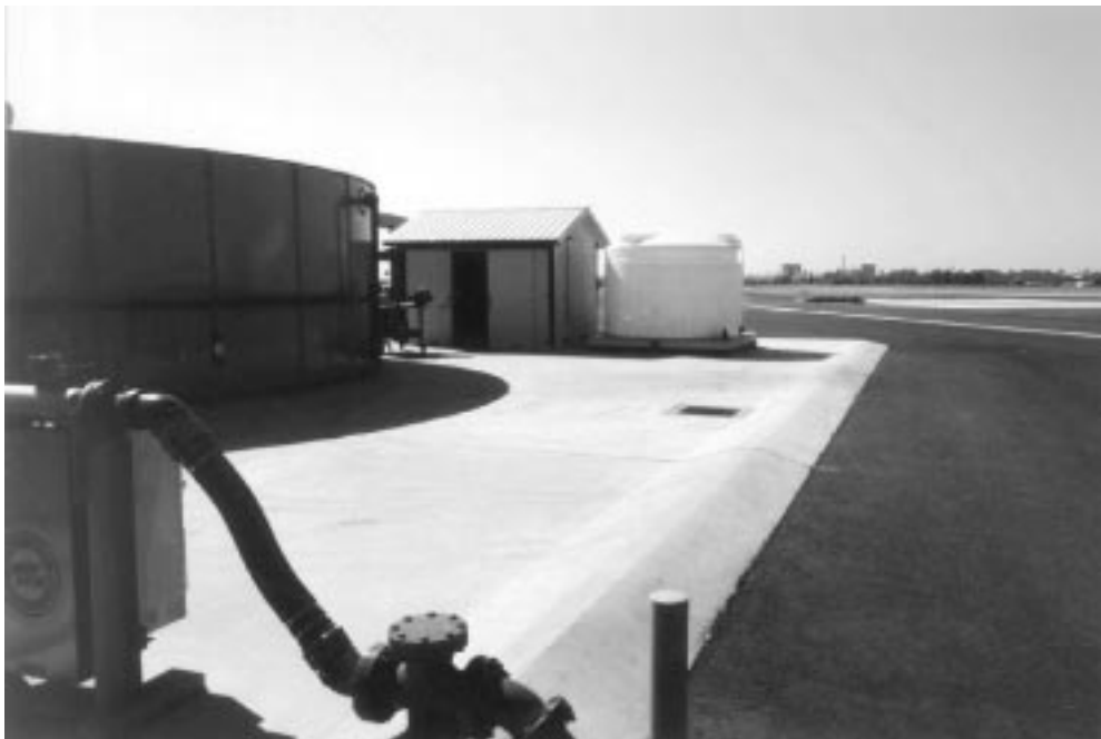
Figure 40. Tank and Service Area Spill Containment Concrete Berm—Fresno, CA. Berm allows for service equipment access to tanks and their associated equipment. This method requires a larger concrete surface (tank pad) to achieve proper spill containment. It is a good idea, if feasible, for all bases to consider.
