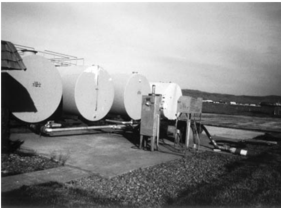
Figure 19. Storage Tank Pad LaGrande, OR.
