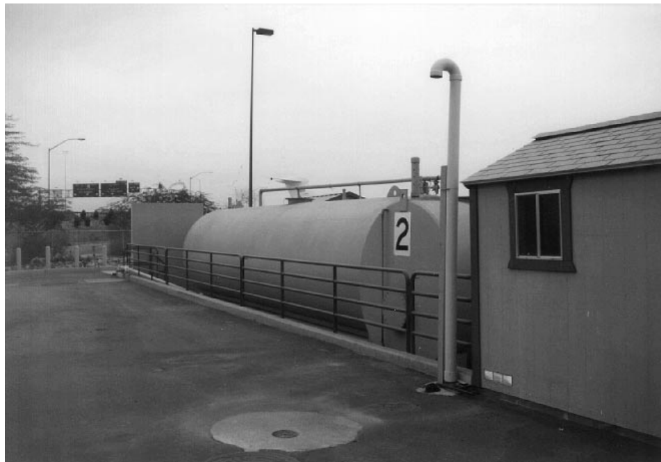
Figures 41 A&B. Tank Spill Containment Pit—Phoenix, AZ.
