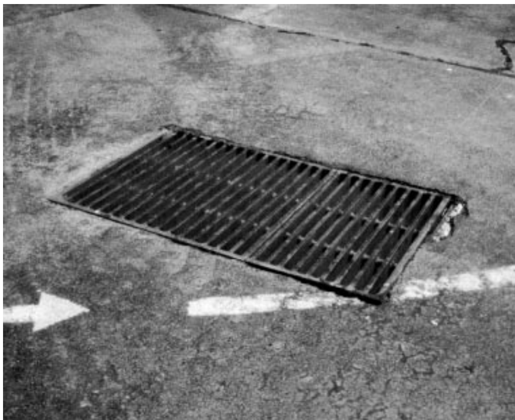
Figure 23. Runway Drain—Klamath Falls, OR.
