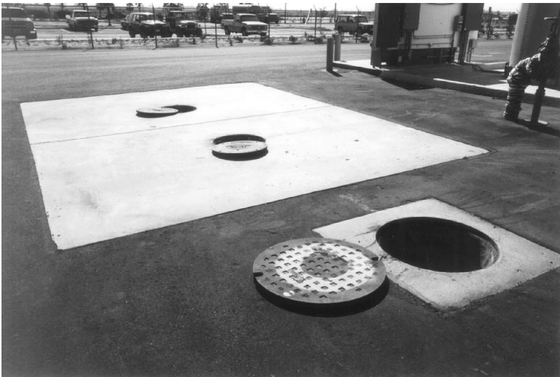
Figure 49. Oil/Sand Separation Tank for Municipal Sewer Connection—Fresno, CA.
