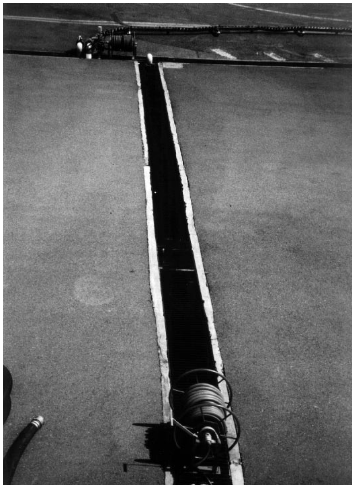
Figures 28 A&B. Tank Pad Drain—Medford, OR.
