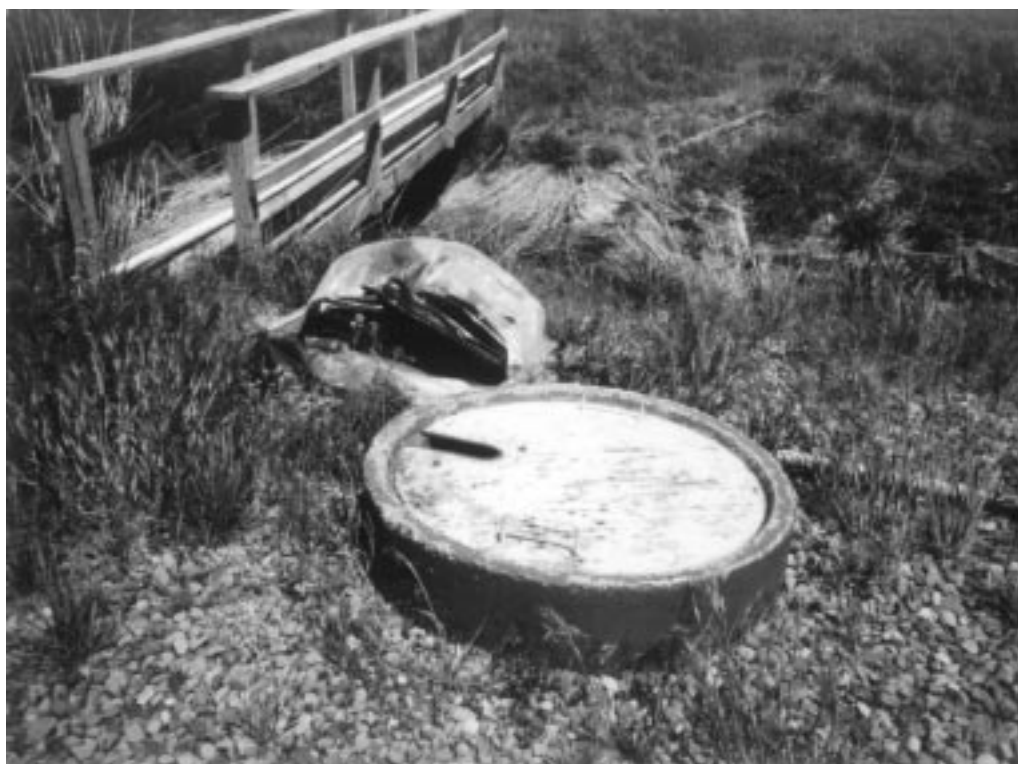
Figure 24. Separation Tank Sump—Klamath Falls, OR.
