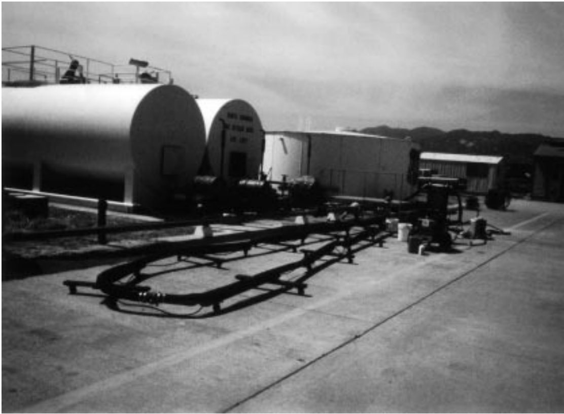
Figure 8. Storage Tanks—Santa Barbara, CA.
