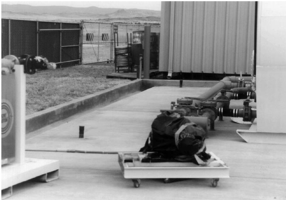
Figures 52 A&B. Storage Tank Spill Isolation Pad—Prescott, AZ.
