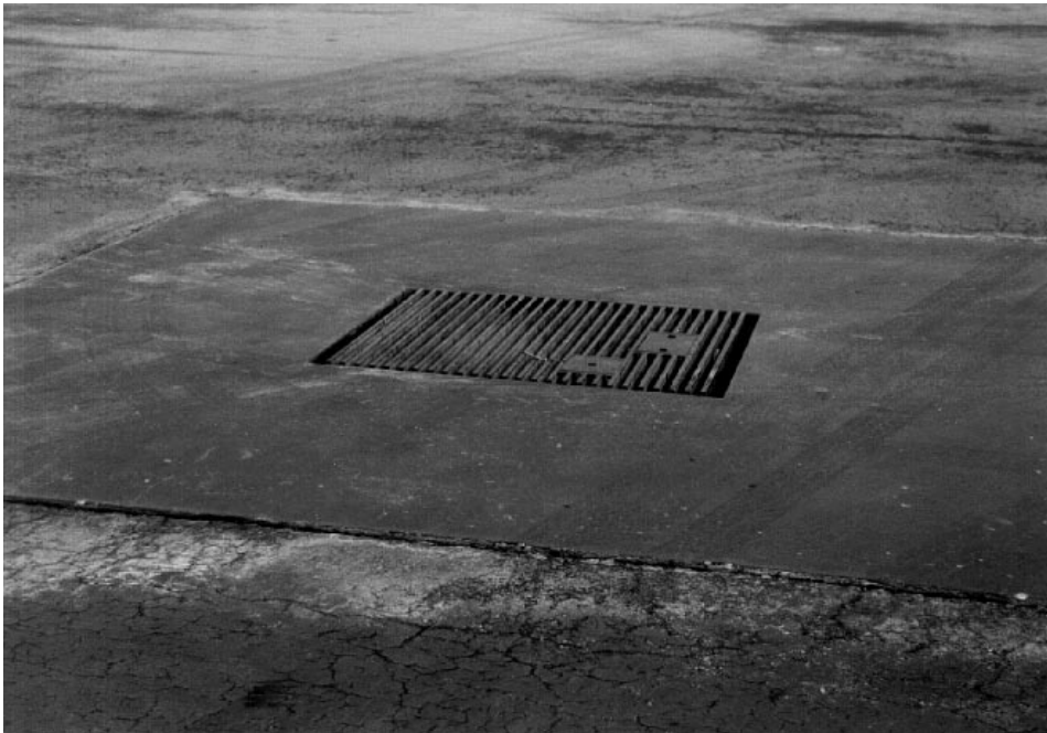
Figure 38. Aircraft Loading Area Drain—Phoenix, AZ.
