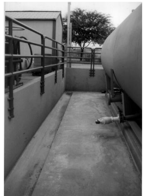
Figure 1. Storage Tank Containment—Phoenix, AZ.
