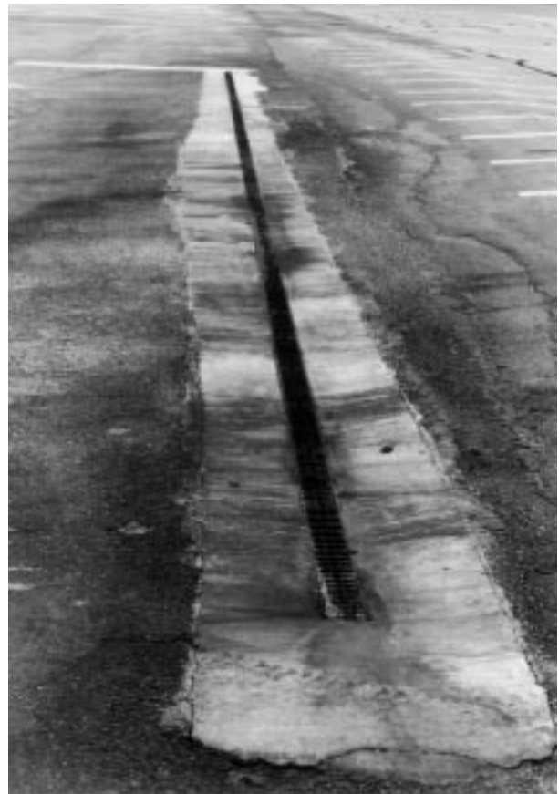
Figure 46. Asphalt Berm with Drain—Wenatchee, WA.
