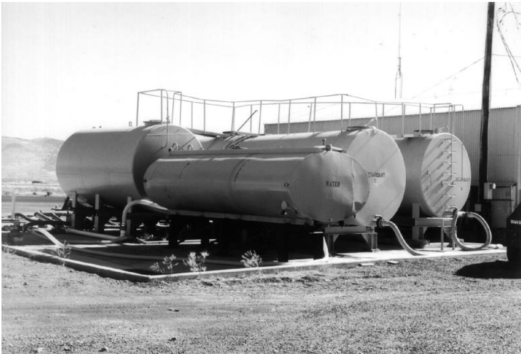
Figure 44. Tank Spill Containment—Lakeview, OR.
