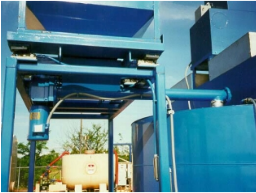
Figure 21a—View of powder conveyor and hopper platform load cells.
