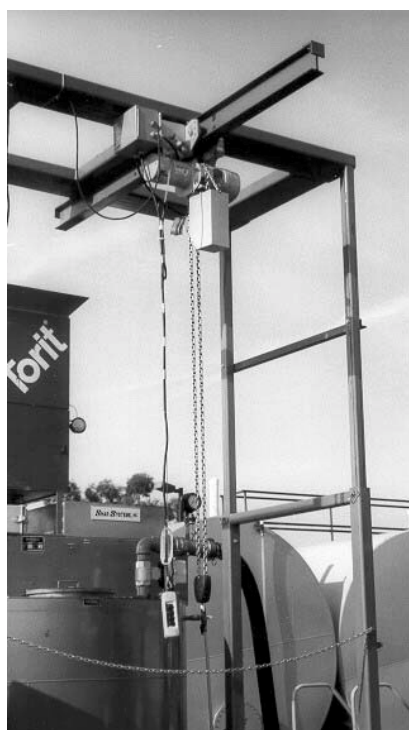
Figure 24—Two-ton hoist and powered trolley assembly.
