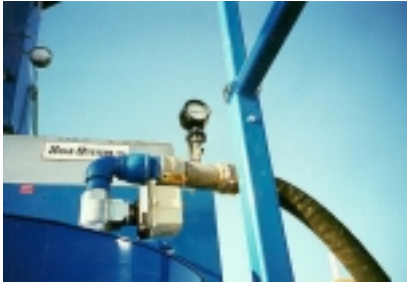
Figure 9a—Mixer water inlet line with 3-inch motor operated ball valve. Connection to base water is with 4-inch camlock fitting.
