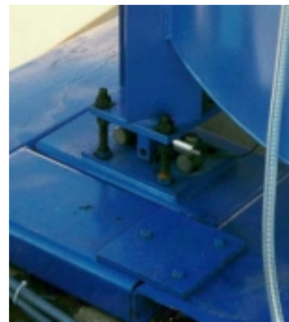
Figure 12—Mixer tank load cell.
