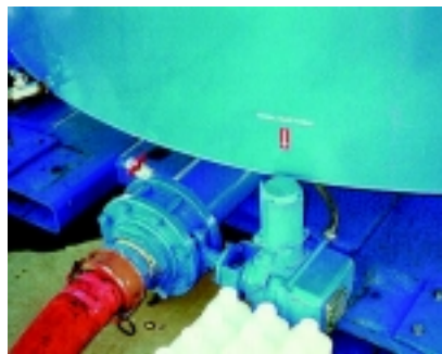
Figure 9b—Mixer outlet connection to transfer pump. Connection is made with 4-inch camlock fitting.
