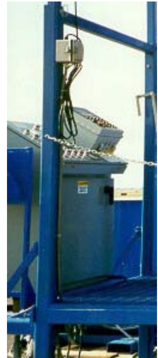
Figure 13—Mixer electrical control console (weather proof enclosure).
