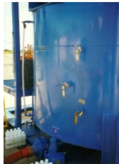
Figure 19—Sampling valves installed on mix tank.
