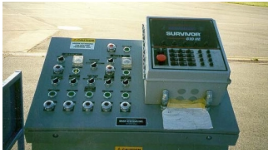
Figure 14—Mixer control panel.
