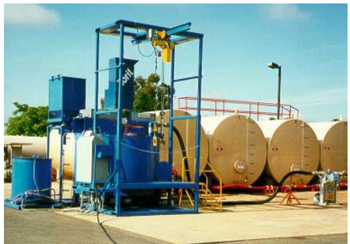
Figure 16—View of mixer system test setup at Redding Airtanker Base.
