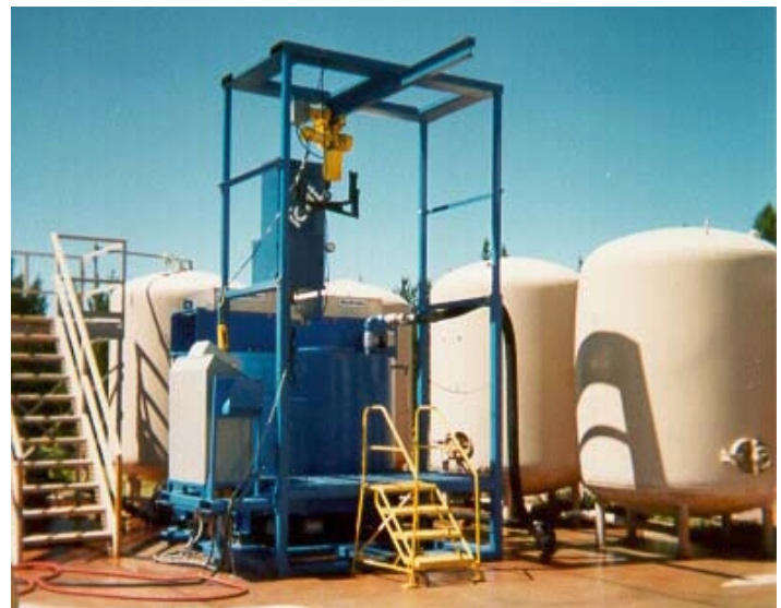
Figure 17—View of mixer system installation at West Yellowstone Airtanker Base.
