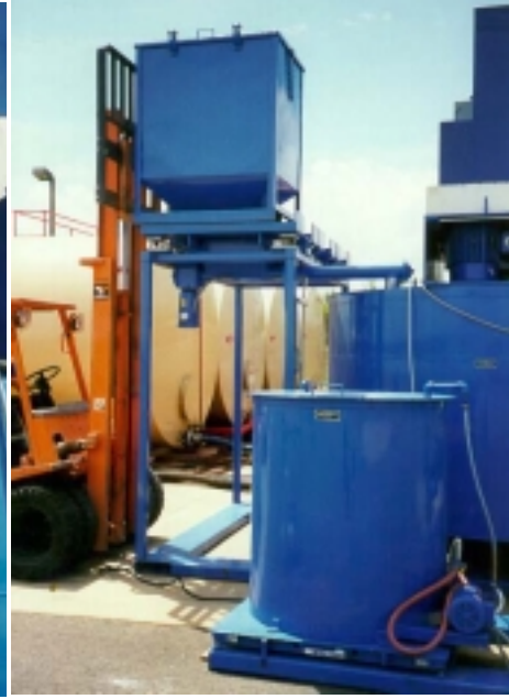
Figure 21b—Positioning powder hopper with fork lift. Notice liquid feed tank in the foreground.
