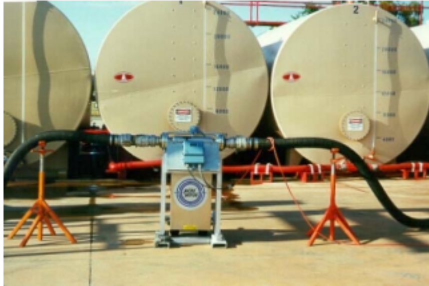
Figure 18—Micro Motion Flowmeter installed in water fill line at Redding Airtanker Base.
