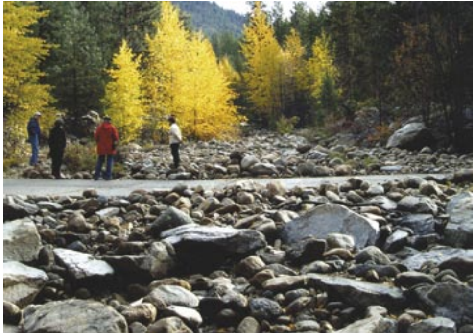
Figure A6—Vented ford plugged with boulders.
