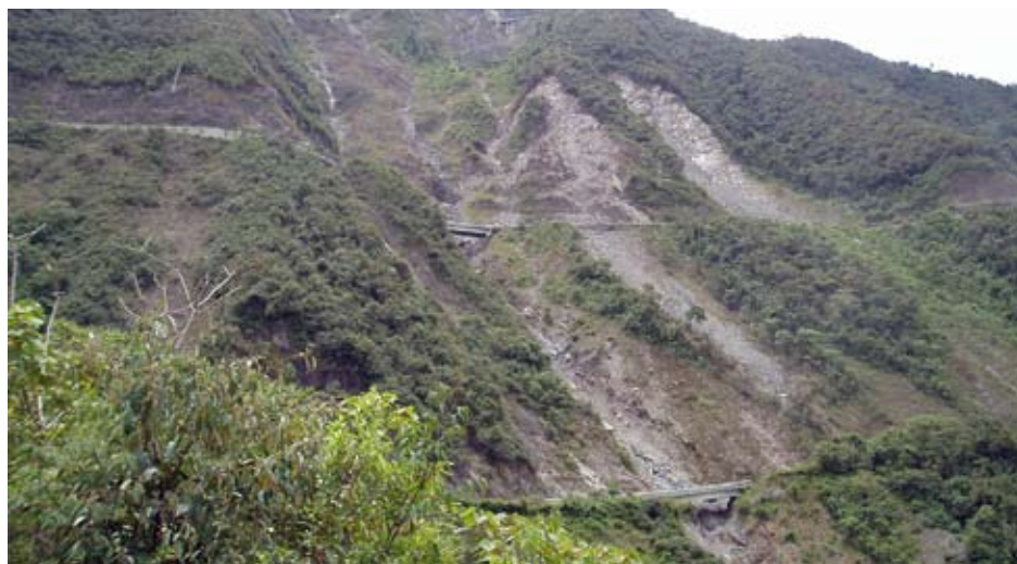
Figure 2.4—Road located on a geologically unstable slope causes massive landslides, Bolivia.
