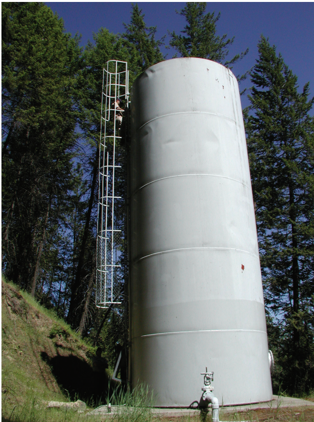
Figure 30—Welded steel water tank.
