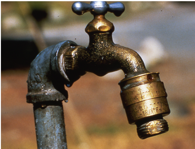
Figure 43—Hose bib with vacuum breaker.
