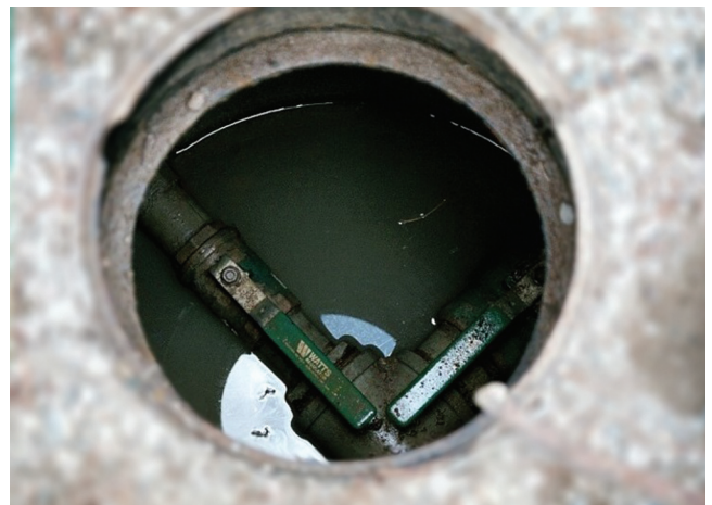
Figure 82—Leaking valve under water.
