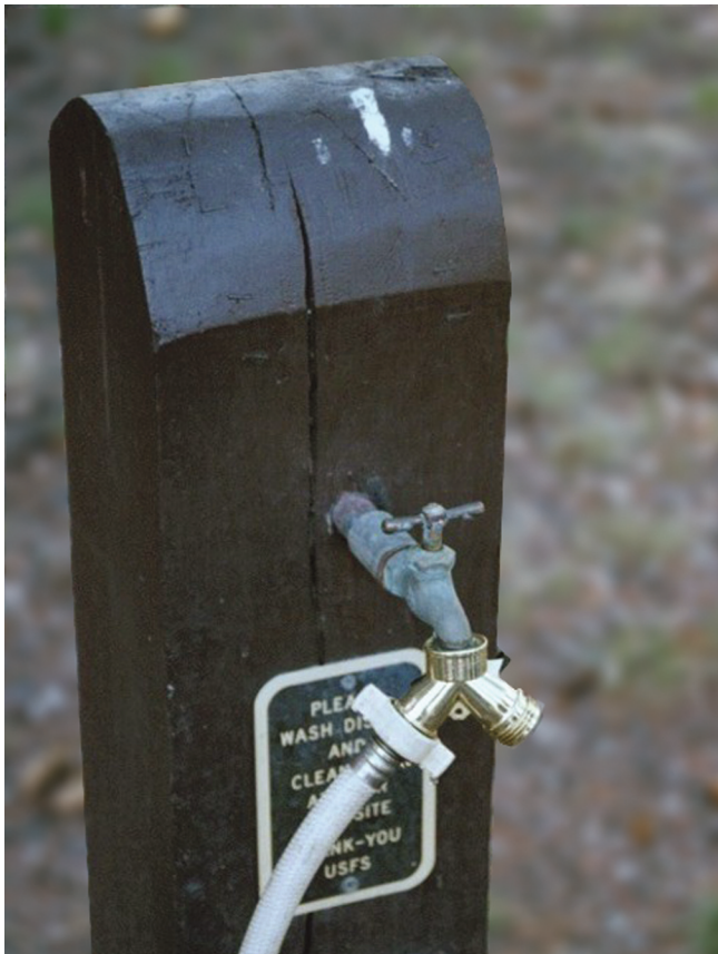
Figure 83—Missing atmospheric vacuum breaker.
