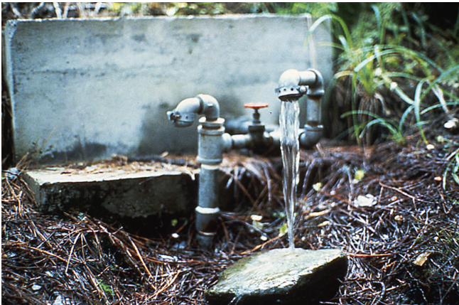
Figure 56—Open winter bypass valve.
