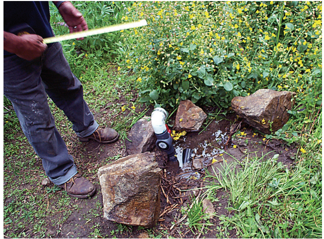
Figure 57—Drain all water lines.
