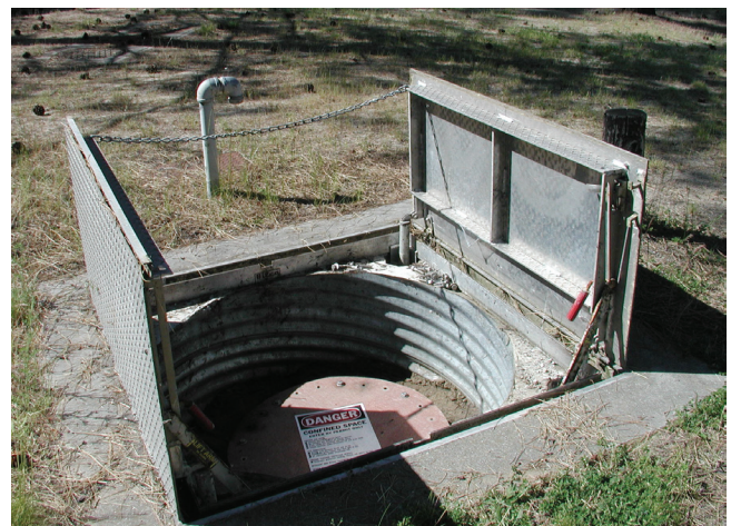
Figure 51—Tanks are confined spaces.
