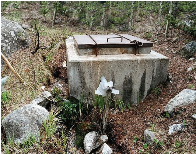
Figure 48—Spring box with erosion damage.
