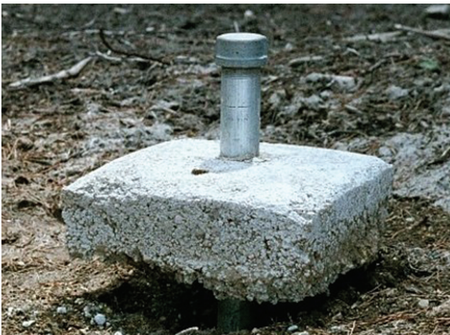
Figure 49—Erosion around vent.
