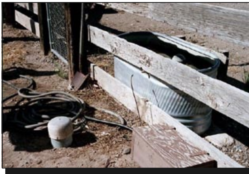
Figure 5—This stock tank water supply is a cross-connection disaster waiting to happen.
