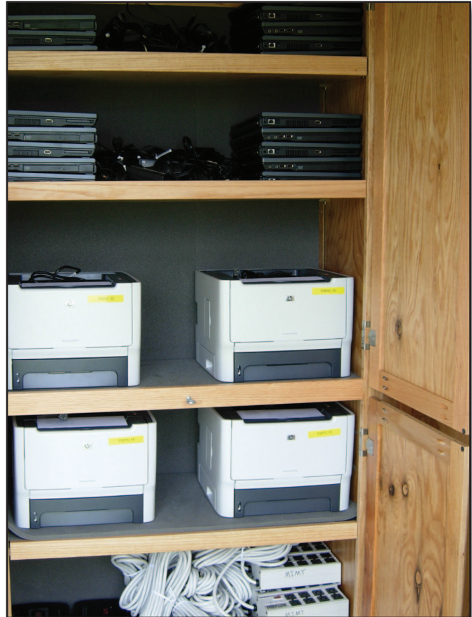
Figure 3—Two large storage cabinets inside the trailer hold the mobile thin clients, printers, and networking hardware.
