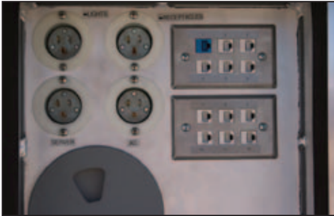
Figure 5—A hatch door on the side of the MIMIT trailer allows access to the power circuits (4) and external networking data ports (12) that connect to network cables at the incident command post.
