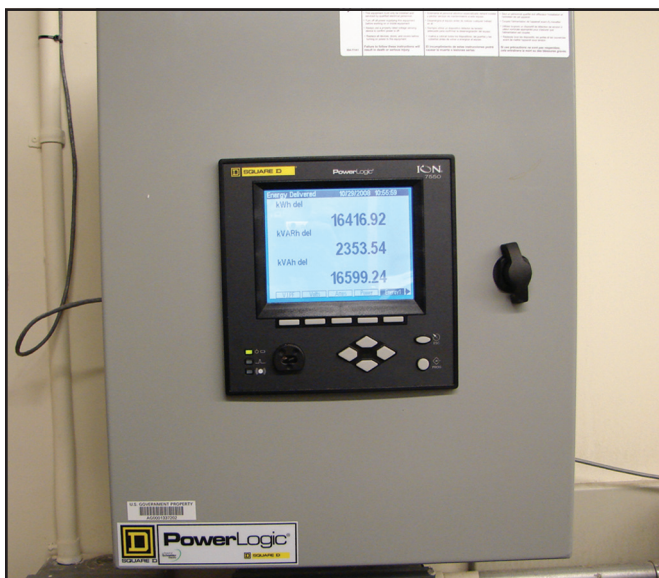
Figure 1—A typical high-end meter suitable for monitoring the electrical feed from an electric utility to a Forest Service facility.
