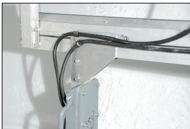
Figure 10e—The electrical cable and electrical wire are routed along the end of the rail.
