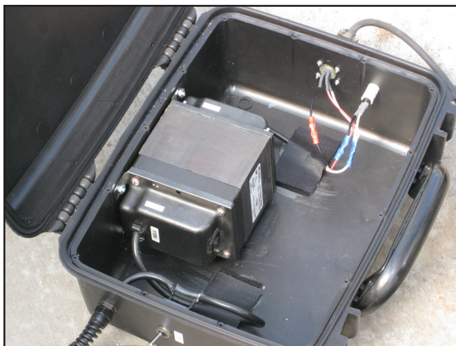
Figure 13a—The voltage transformer.
