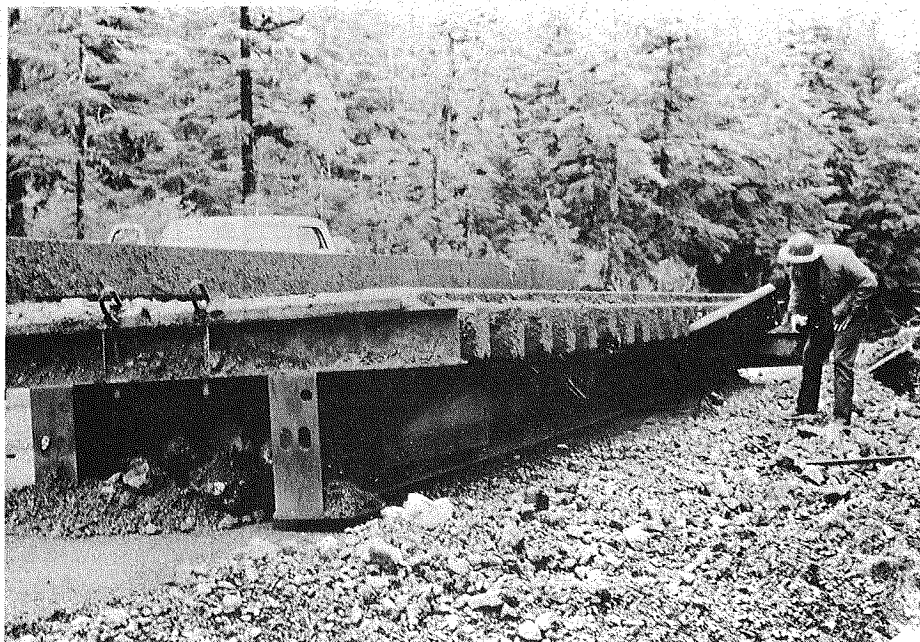
Figure 14.--Slight damage sustained while skidding the bridge section up the road during emergency removal. The front end of the bridge dug into the roadway surface on curves. The damage was easily repaired and the bridge was returned to service.
