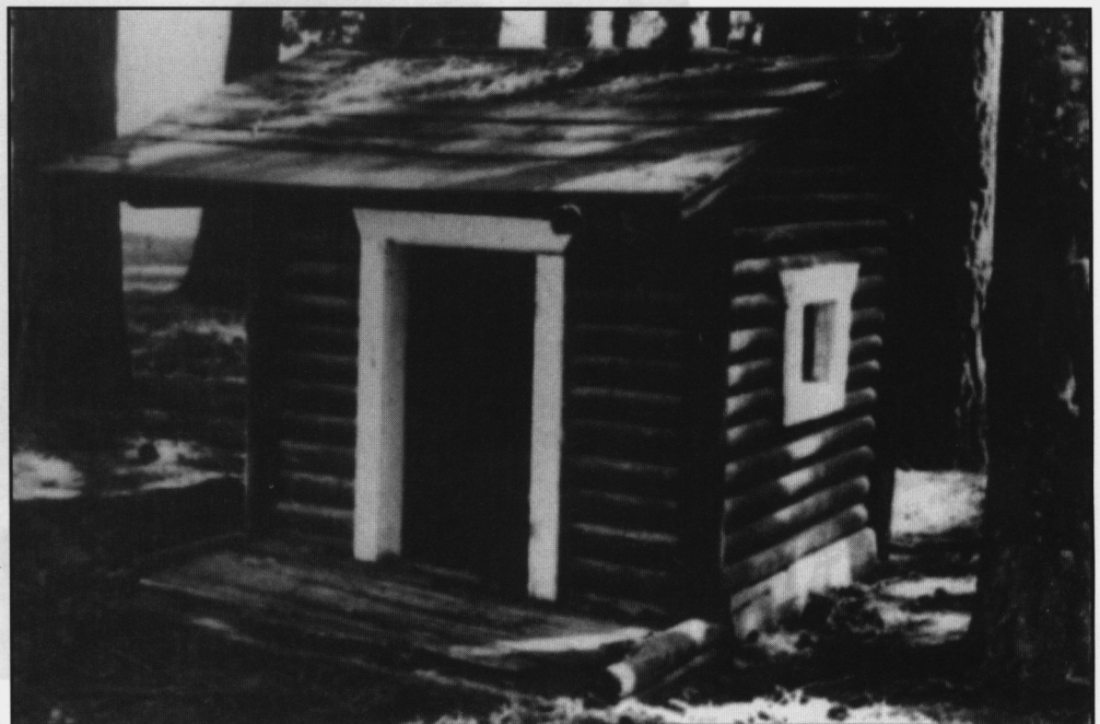
Figure 2. Vierhus Playhouse in disrepair
