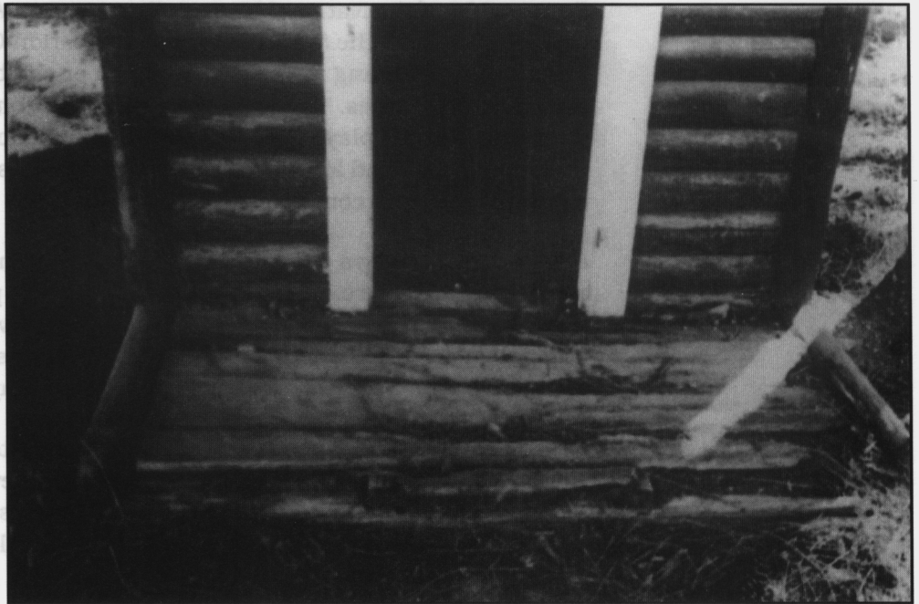
Figure 3. Rotted sill logs
