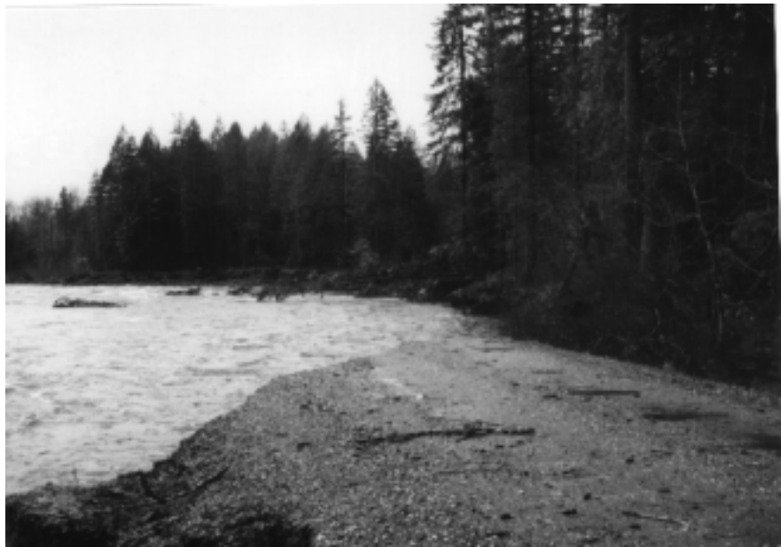
Figure 7. Suiattle River scours about a quarter mile of road.
