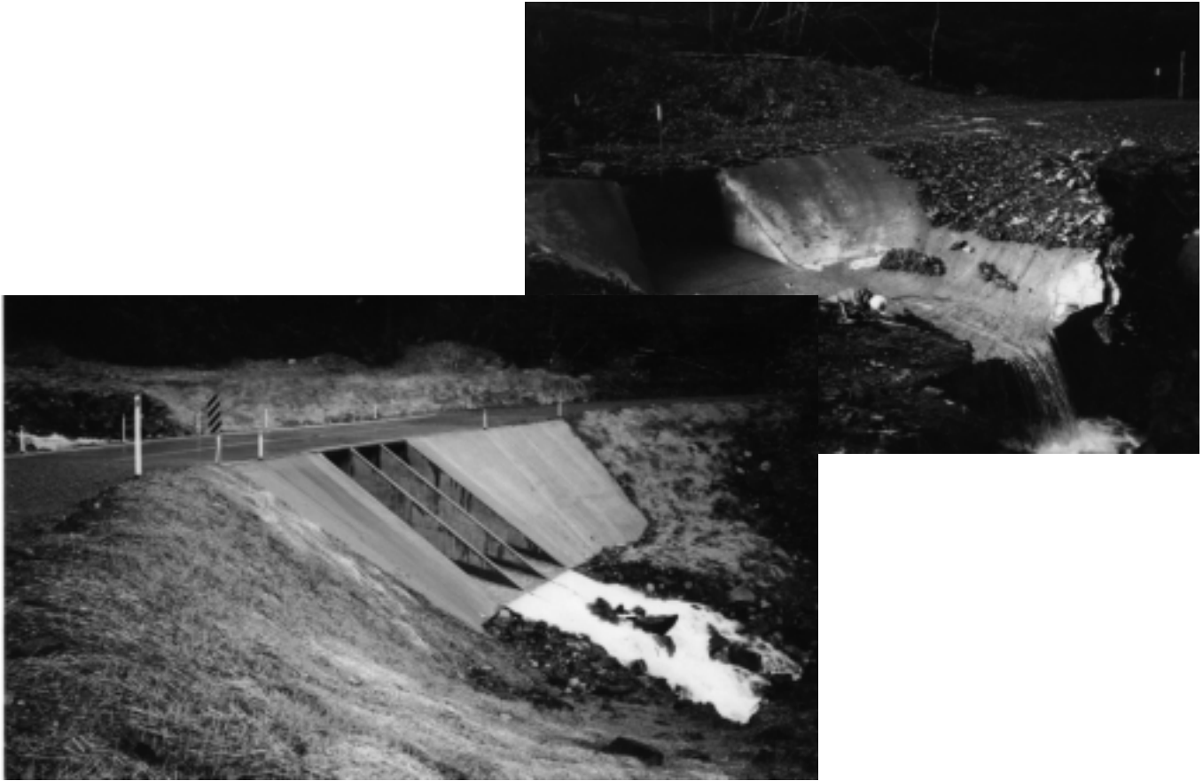
Figure 11. A ford follows a storm, with debris on the surface and minor damage at the outlet (upper-right photo). Subsequent designs include large riprap at the outfall as an energy dissipator (lower-left photo).
