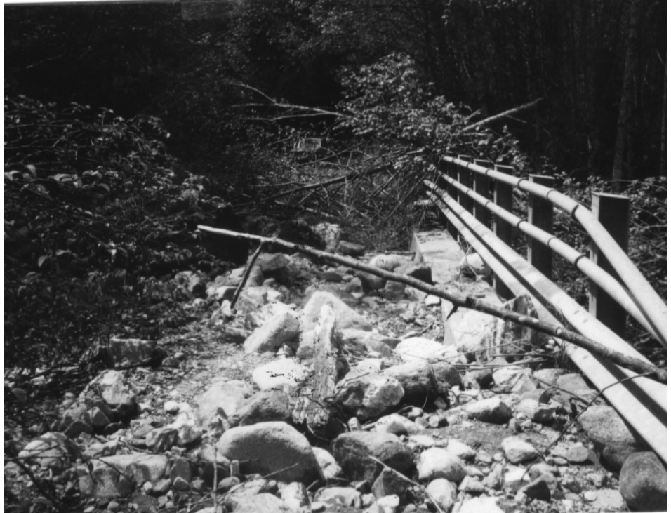
Figure 8. Bedal Creek flows over the top of a bridge.
