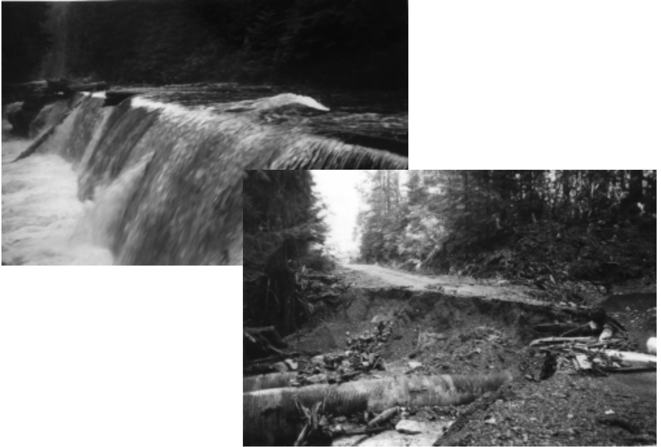
Figure 10. Providing cross drainage for major streams is a challenge due to high energy and debris flow.
