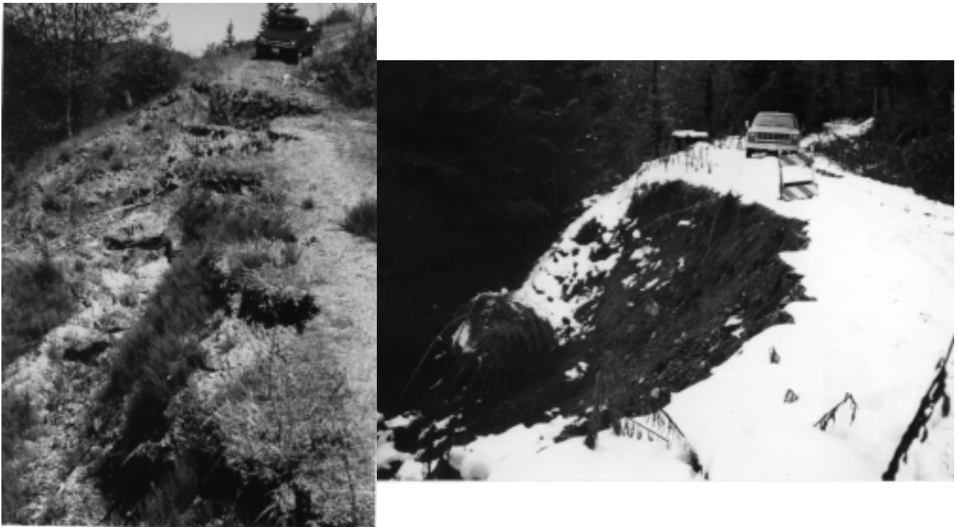
Figure 12. Slumping and side-cast failures are typical along hundreds of miles of local road on the forest.
