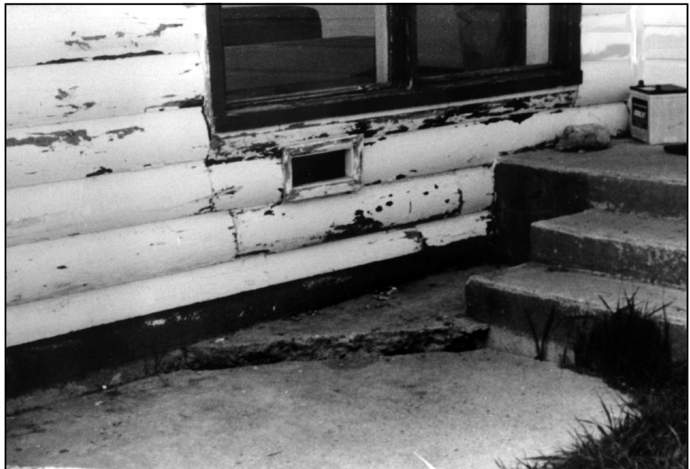
Figure 9. Unsafe sidewalk at bunkhouse.
