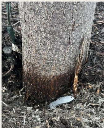
A pocketknife is used to show the excessive mulch piled near the base of this tree.
