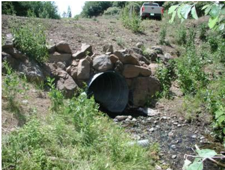
Figure 87. Culvert replaced on Fourth of July Creek. Photograph is looking downstream at the inlet of the culvert in July 2008.
