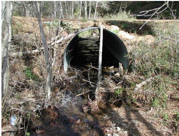
Figure 73. Culvert replaced on Adams Creek. Photograph is looking upstream at the outlet of the culvert in the spring of 2007.
