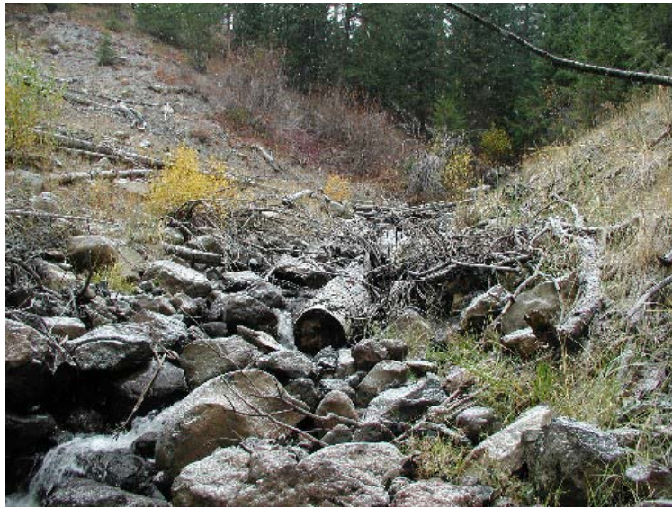
Figure 65. Culvert removal on Bull Corral Creek. Photograph is looking upstream at the culvert location in October of 2007.
