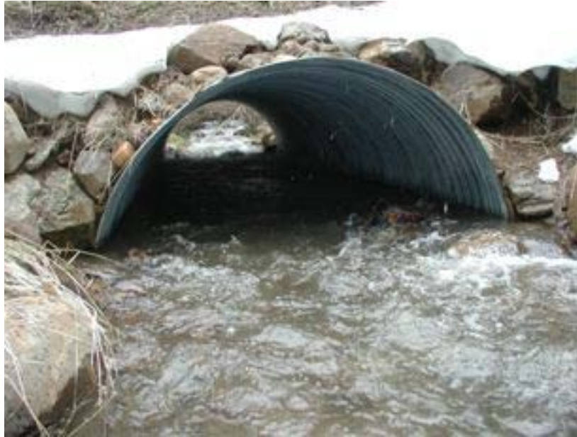
Figure 16. Outlet of the culvert on FS Road 110 (unnamed tributary of Bear Creek) on May 21, 2008.
