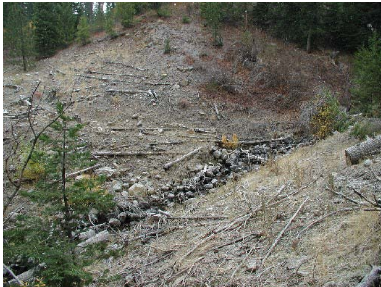
Figure 66. Culvert removal on Bull Corral Creek. Photograph is looking upstream at the culvert location in October of 2007.
