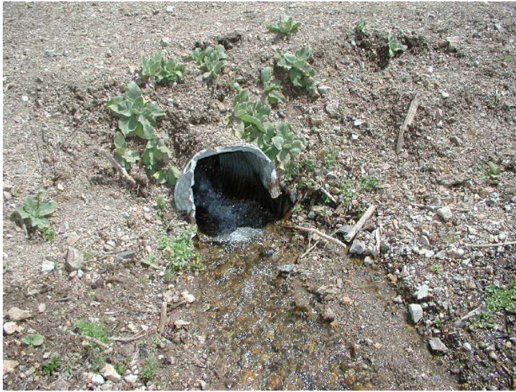
Figure 94. Culvert on Barton Gulch, looking at the bent inlet in the spring of 2007.
