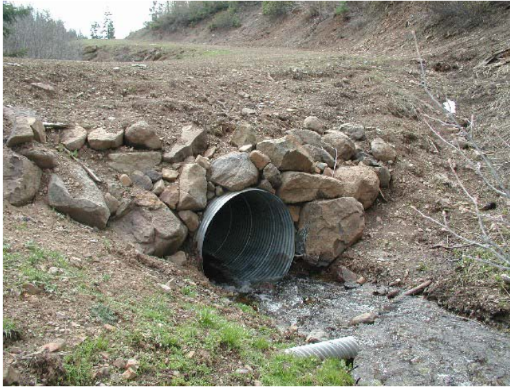
Figure 84. Culvert replaced on Fourth of July Creek. Photograph is looking downstream at the inlet of the culvert in the spring of 2007.
