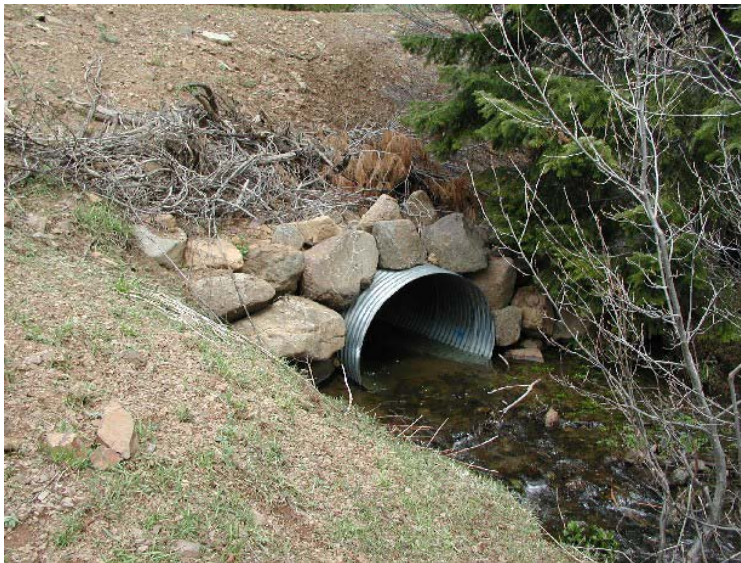
Figure 85. Culvert replaced on Fourth of July Creek. Photograph is looking upstream at the outlet from the left bank.
