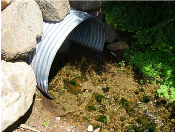
Figure 92. Culvert outlet on Fourth of July Creek. Photograph is looking at outlet pool in June 2009.
