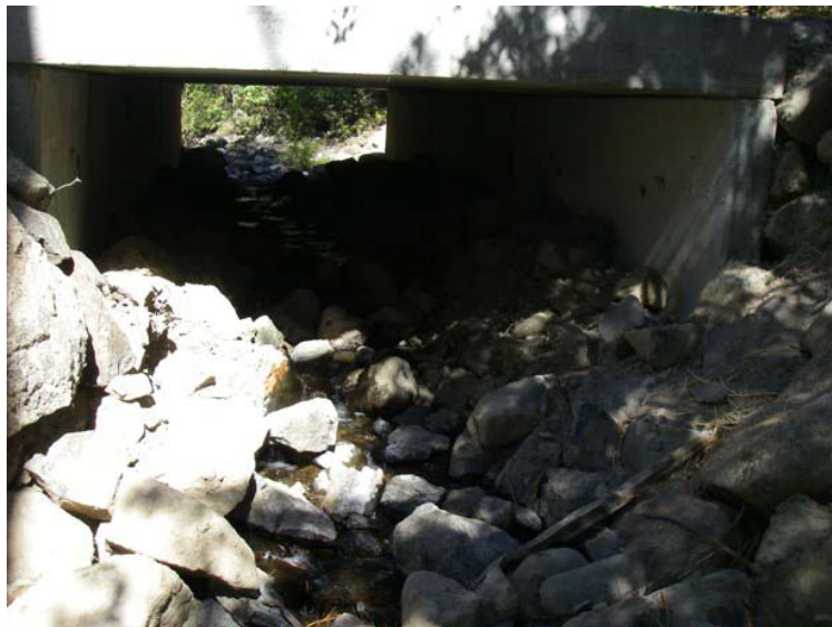
Figure 127. Bridge installed on Boulder Creek. Looking upstream at the outlet of the bridge on September 23, 2009.
