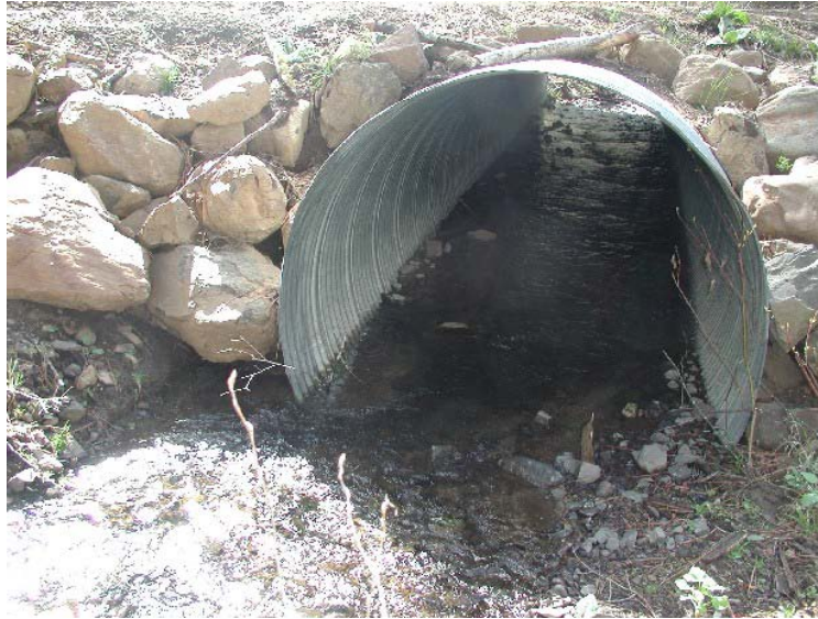
Figure 72. Culvert replaced on Adams Creek. Photograph is looking downstream at the inlet of the culvert in the spring of 2007.
