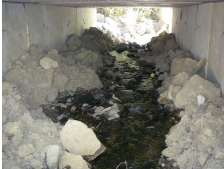
Figure 128. Bridge installed on Boulder Creek. Looking downstream at the channel inside the bridge on September 23, 2009.
