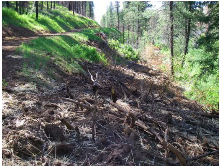
Figure 137. Road decommissioning where the re-route ends at the upstream end on FS 217.
