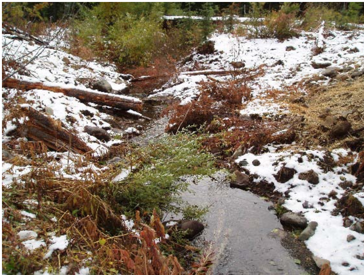
Figure 60. Culvert removal location on an unnamed tributary of Bear Creek on October 2, 2007. Looking downstream.
