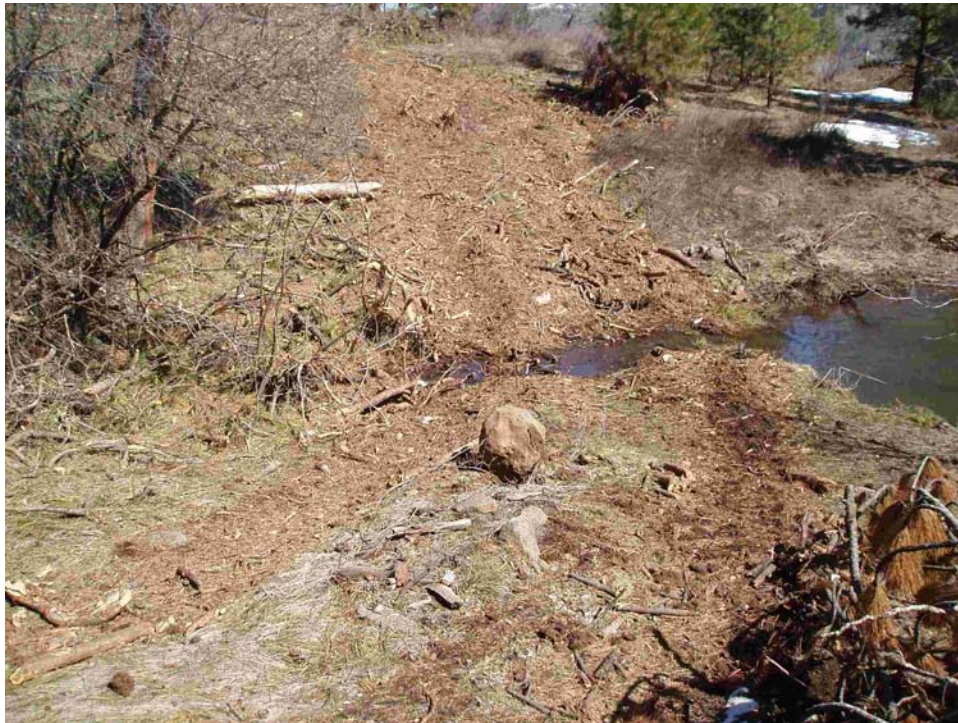
Figure 17. Intermittent channel where snow bridge was located in unit 5 of Bear West after snow melt. Pool on right side of photograph is part of the Bear Irrigation Ditch, which captures the channel. See Figure 16 for pre-snow melt photograph.
