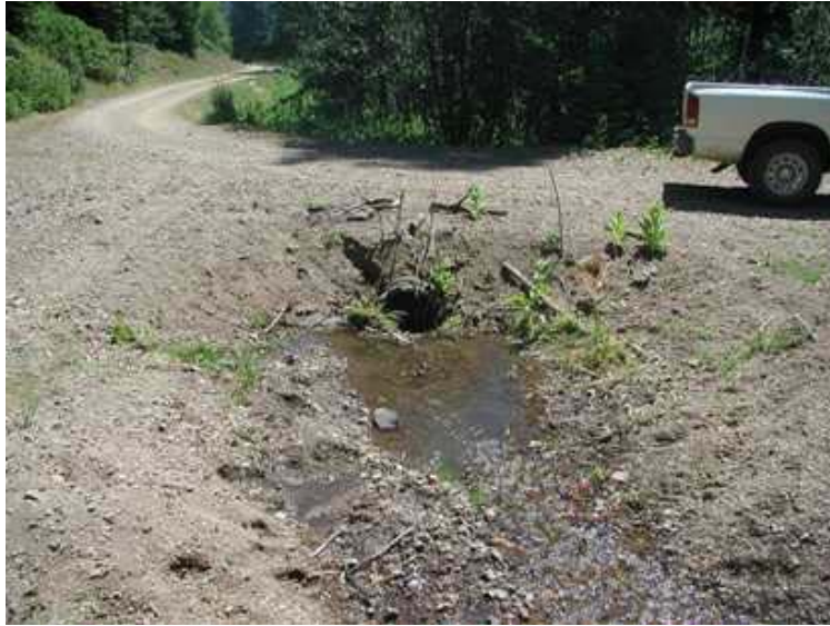
Figure 96. Culvert on Barton Gulch, looking downstream at the inlet in the spring of 2008.
