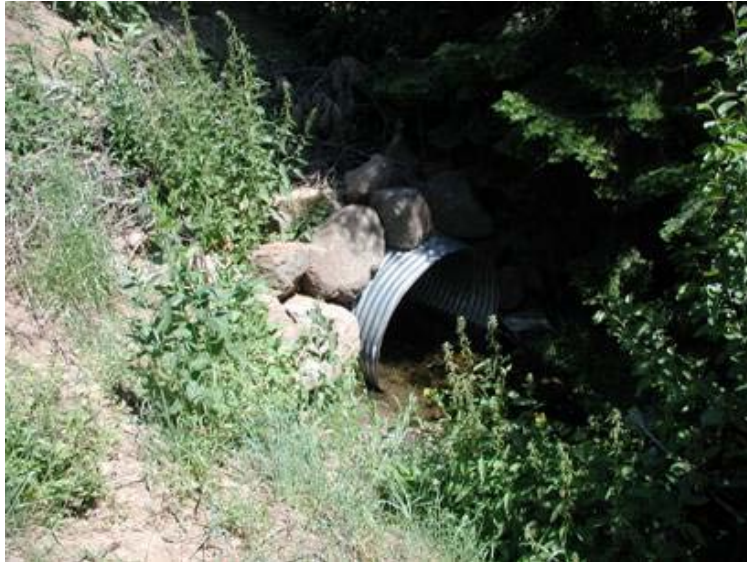
Figure 88. Culvert replaced on Fourth of July Creek. Photograph is looking upstream at the outlet from the left bank in July 2008.
