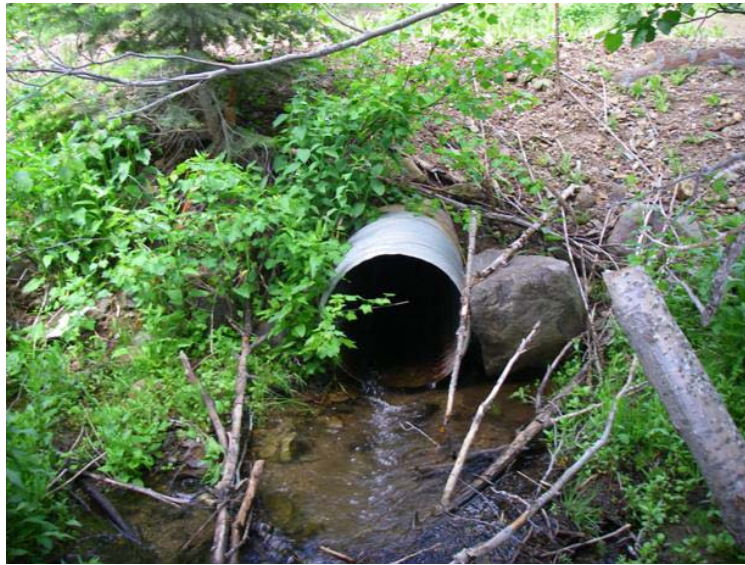
Figure100. Culvert on Barton Gulch, looking upstream at the outlet in the spring of 2009.
