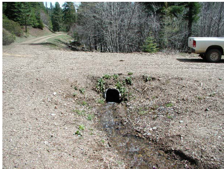
Figure 93. Culvert on Barton Gulch, looking downstream at the inlet in the spring of 2007.
