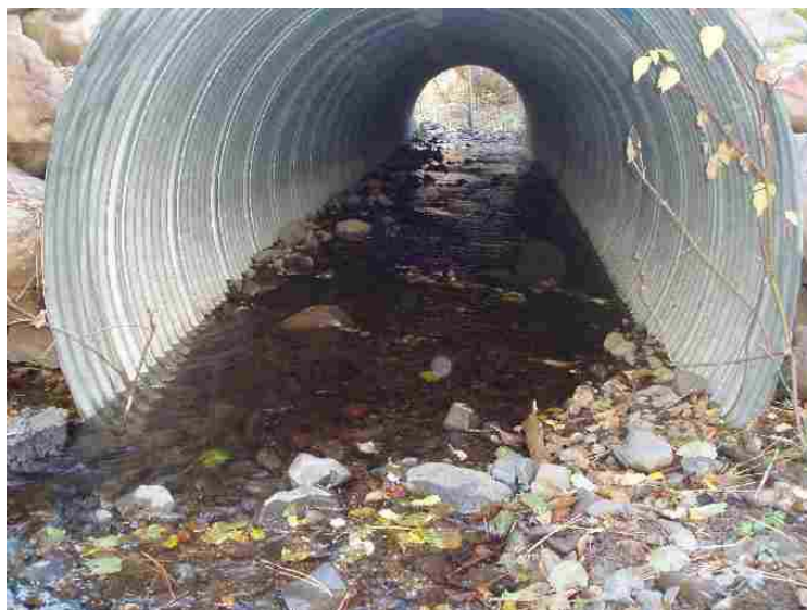
Figure 71. Culvert replaced on Adams Creek to allow fish passage. Photograph is looking downstream at the inlet of the culvert in the fall of 2006.
