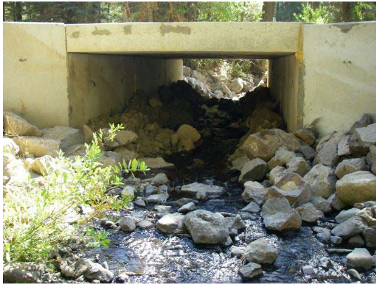
Figure 126. Bridge installed on Boulder Creek. Looking downstream at the inlet on September 23, 2009.
