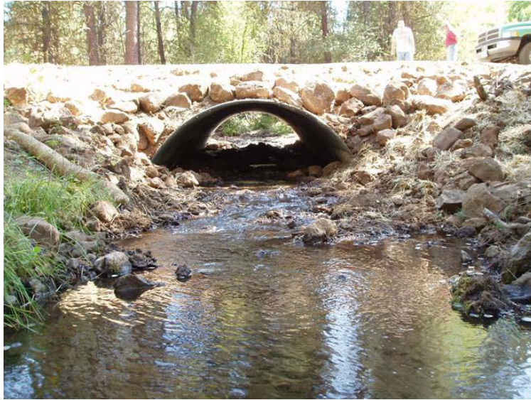
Figure 119. Culvert on FS Road 143 at the Fawn Creek crossing, looking at the outlet after replacement.
