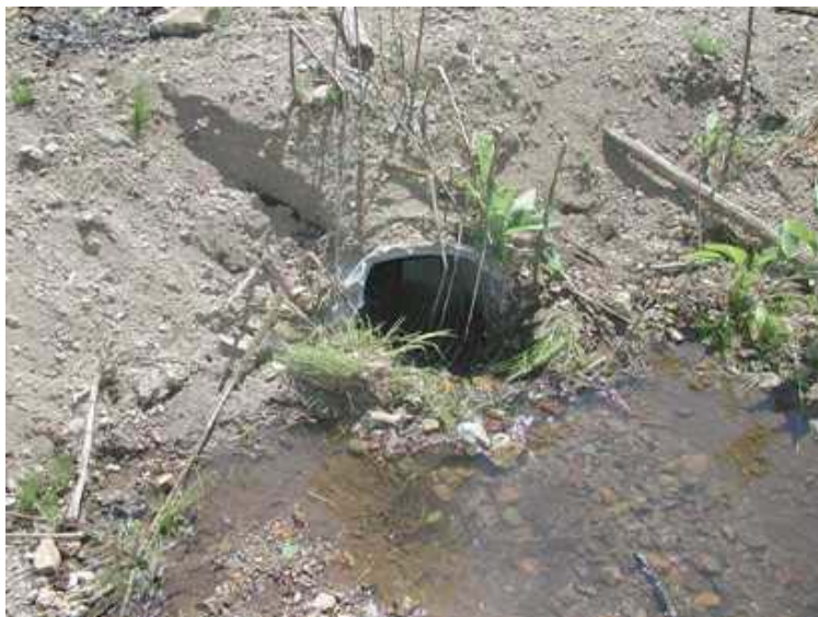
Figure 97. Culvert on Barton Gulch, looking at the bent inlet in the spring of 2008.
