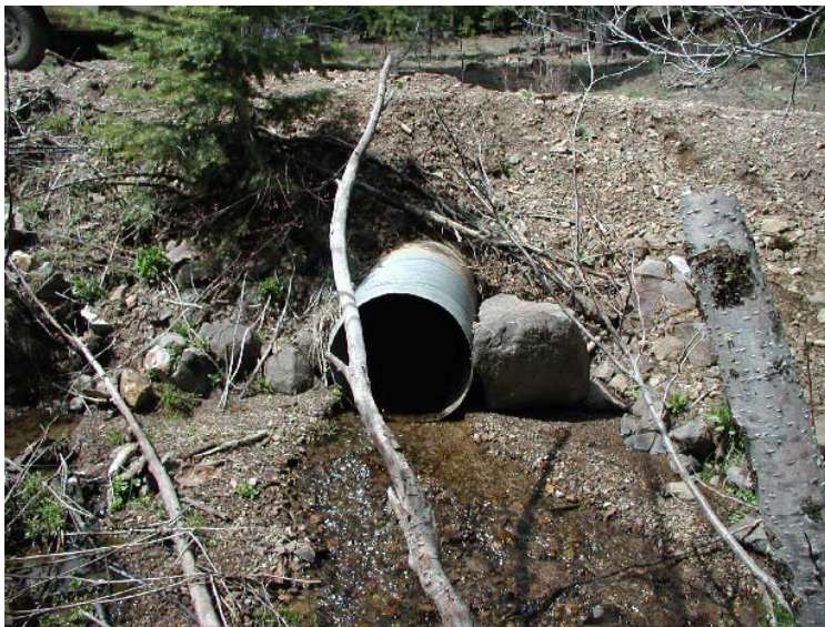
Figure 95. Culvert on Barton Gulch, looking upstream at the outlet in the spring of 2007.
