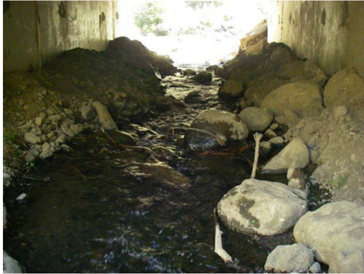
Figure 122. Bridge installed on Warm Springs Creek. Looking downstream at the channel inside the bridge on September 23, 2009.
