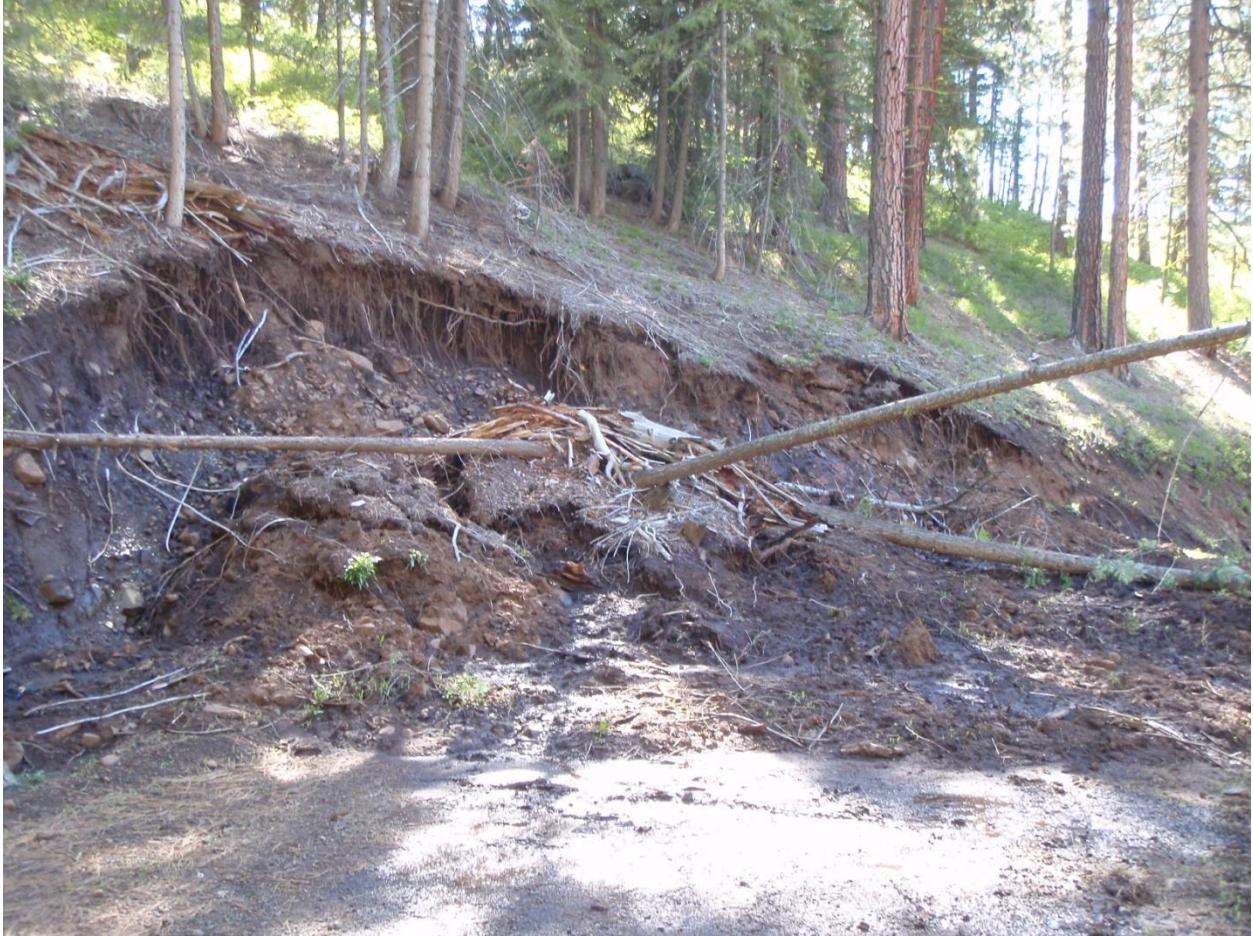
Figure 11: Cutslope failure along control road 50029/50473/50007?.
