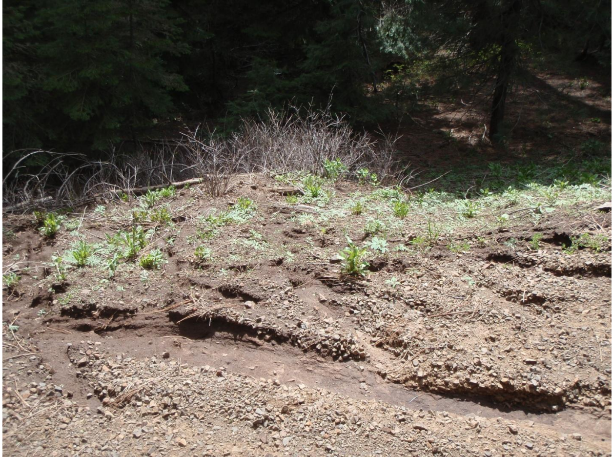
Figure 10: Gully and rills along control road. These extend from the road surface across the fill and onto the hillside below.
