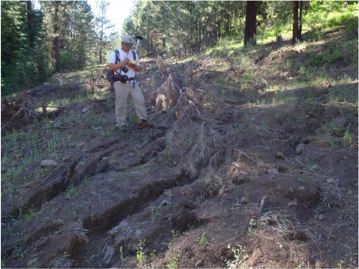
Figure 5: Rills and small gullies on the recontoured road surface.
