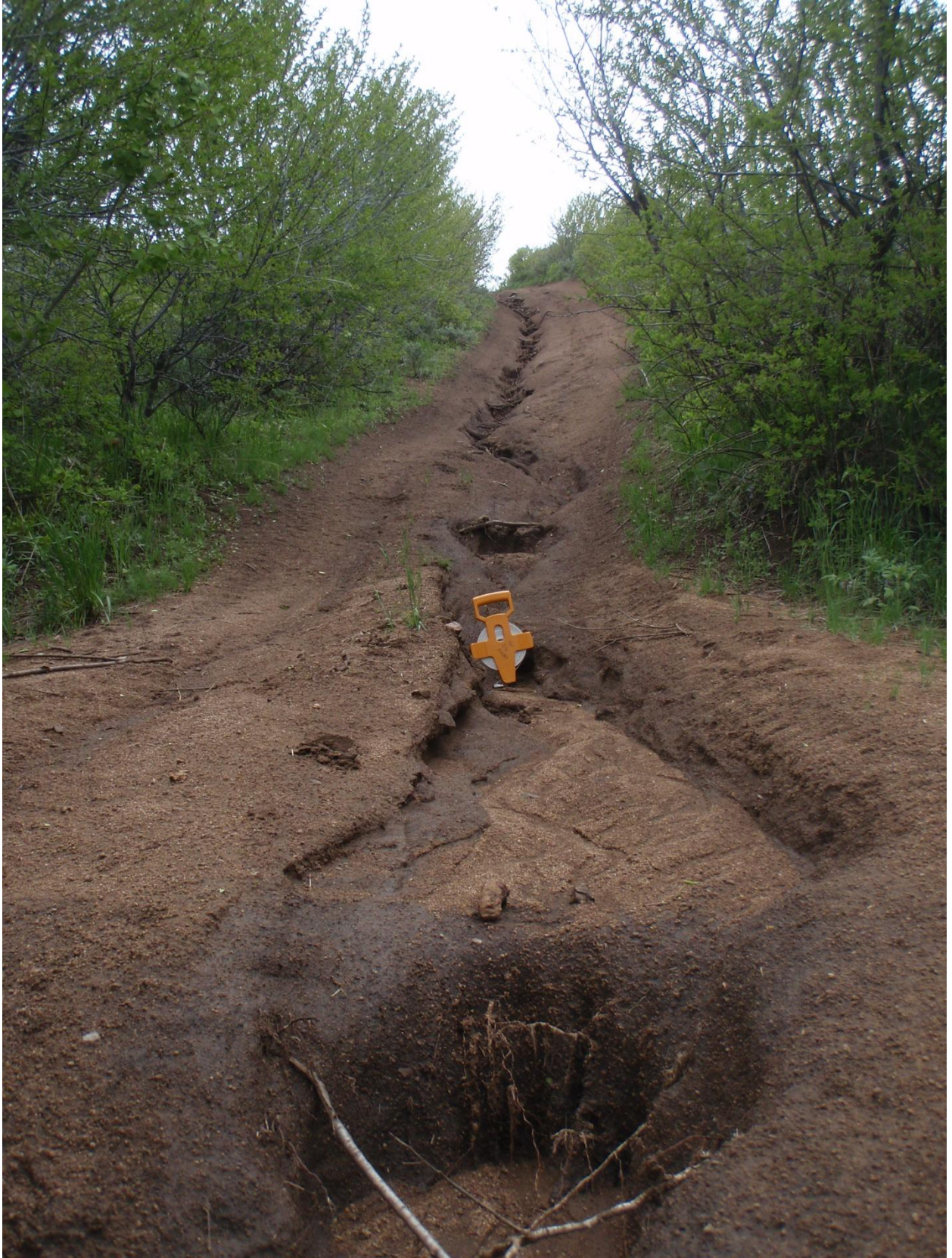
Figure 8: Gullied flowpath on control road 500100500.
