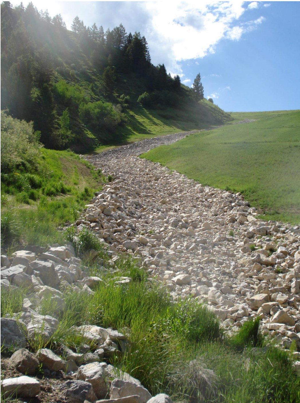
Picture 5 (facing southeast): Down-chute of the SMCM CVF that routes water from the top deck and toe of the dump down and into Maybe Creek just below the outfall. It was noted that the down-chute was damaged last year from water leaving the top deck too quickly moving some of the rip rap out down the chute. Repairs to the down-chute were successful and future potential damage will be mitigated by check dam improvements made in 2021.
