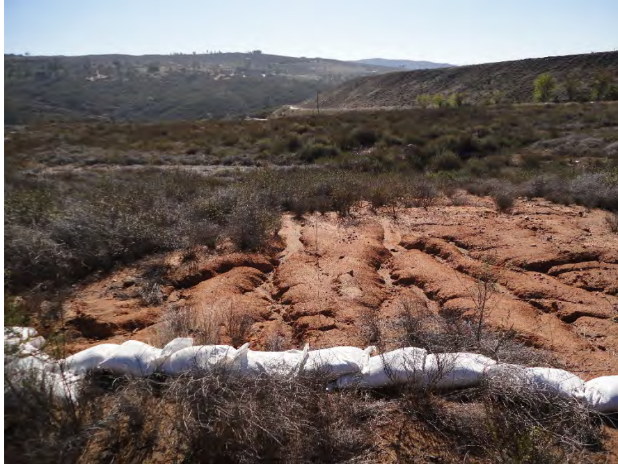
Photograph A-5: View southeast of Site from headwall of erosion scarp. Engineering Evaluation/Cost Analysis, Cleveland National Forest, Ramona, California
