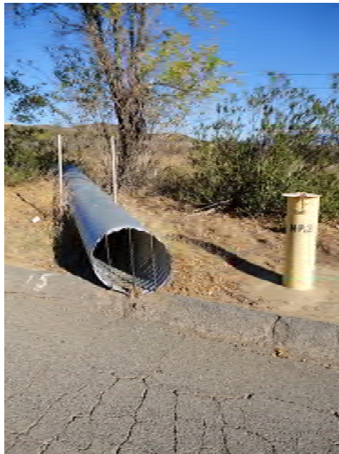
Photograph A-14: View north. Culvert empties onto Dump Road, away from former Burn Dump Site. Engineering Evaluation/Cost Analysis, Cleveland National Forest, Ramona, California Photographed by: Annica Nord (ERRG) Date: October 22, 2013
