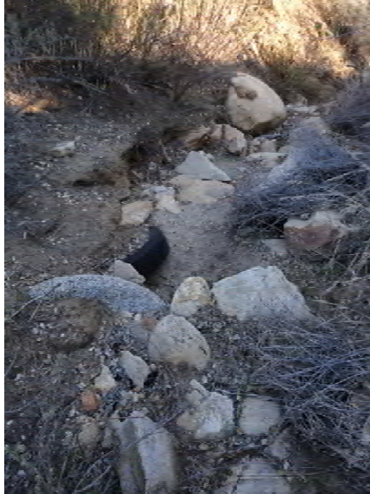
Photograph A-11: Debris in drainage. Engineering Evaluation/Cost Analysis, Cleveland National Forest, Ramona, California Photographed by: Annica Nord (ERRG) Date: October 22, 2013
