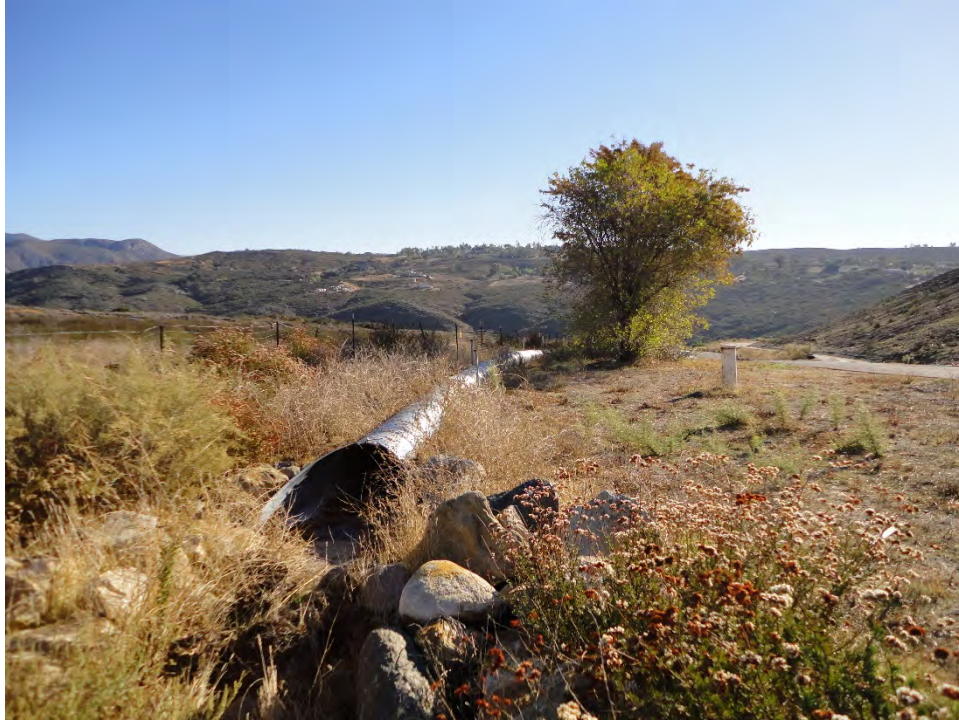
Photograph A-13: View west of culvert installed south of Forest Service property boundary. Engineering Evaluation/Cost Analysis, Cleveland National Forest, Ramona, California Photographed by: Annica Nord (ERRG) Date: October 22, 2013
