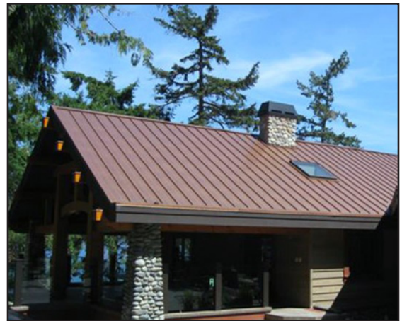
Metal roof—not acceptable
