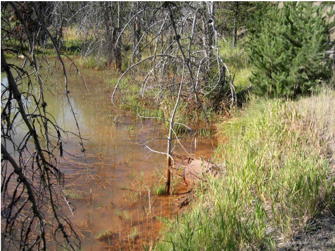
Redboy minewater entering road culvert to Forest Service land.
