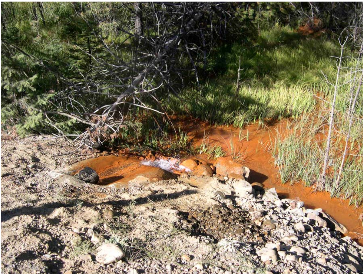
Bluebird discharge pipe.
